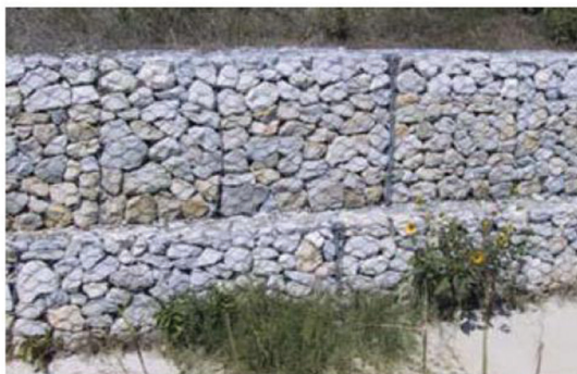
Figure 6.73d Gabions showing a neat, compact, placement of stone with a uniform appearance
