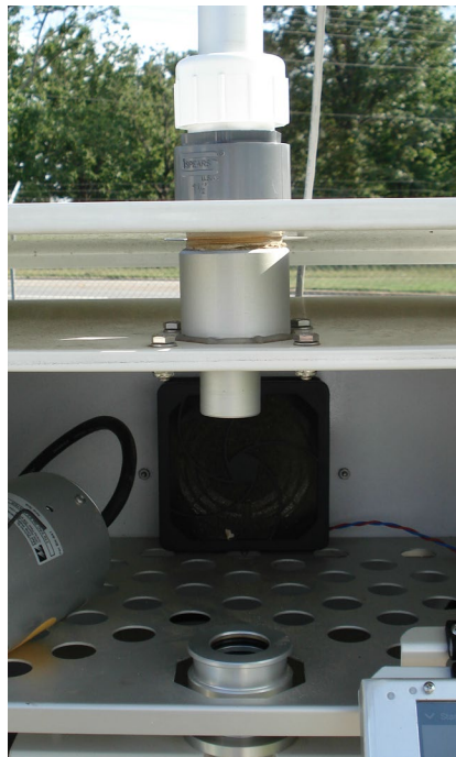
Figure 63. Sample Tube Held in Place by Flange.
