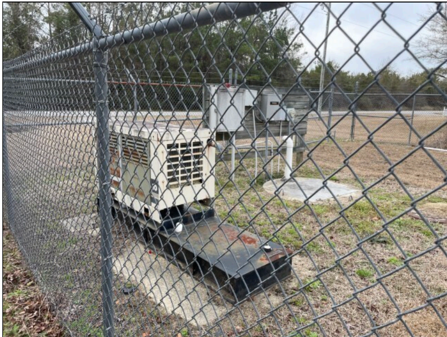
4 - View of lift station on the southwestern portion
