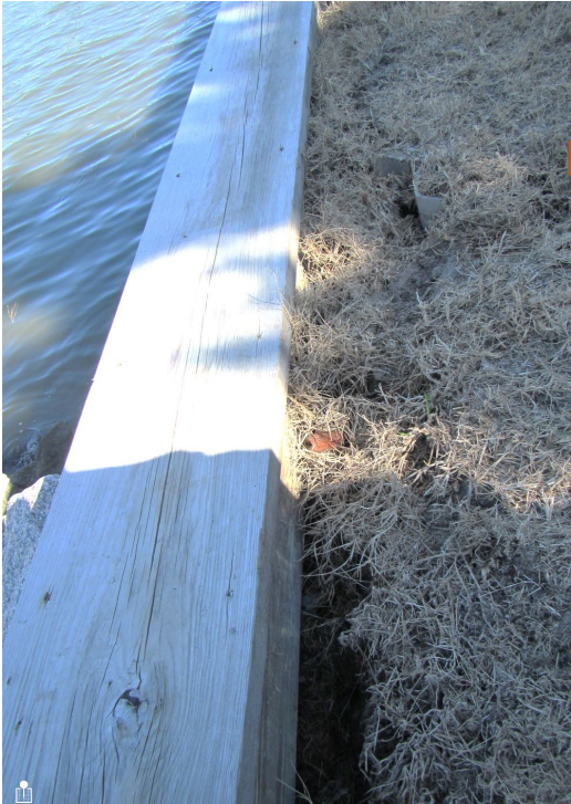
Scour landward of the wall
