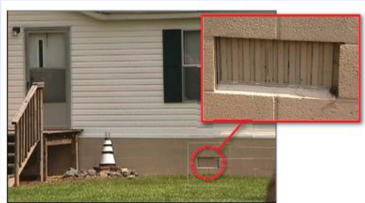
Figure 17: Standard air vent that is unacceptable as a flood opening because it is not disabled in the open position
