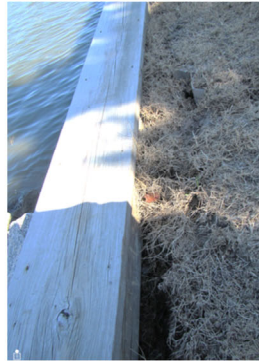
Scour landward of the wall
