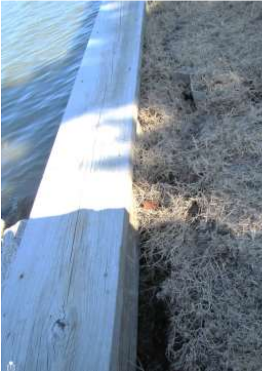
Scour landward of the wall
