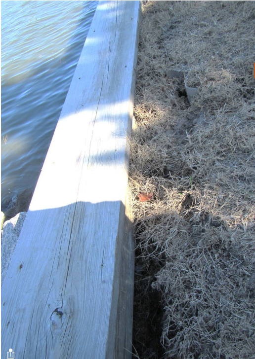
Scour landward of the wall
