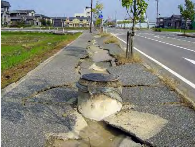
Picture: Manhole breaches pavement as a result of liquefaction
