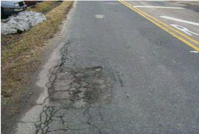
Picture: An example of roadway damage.
