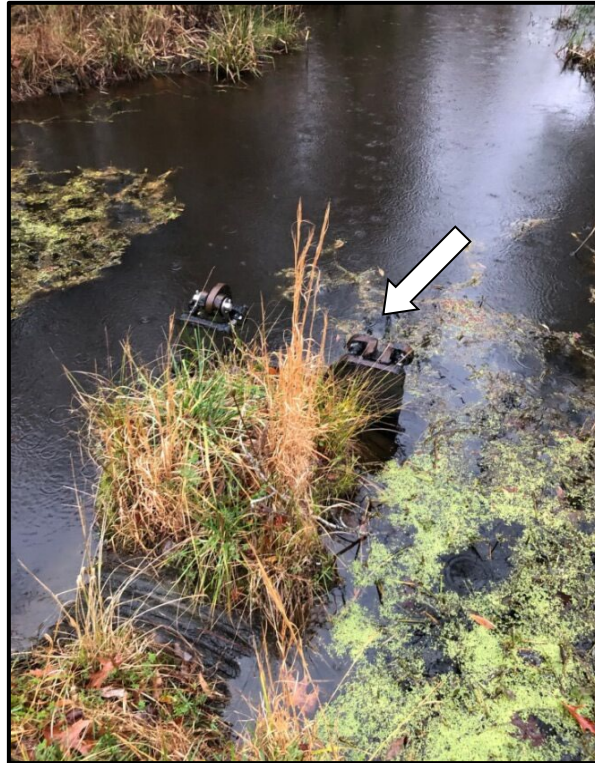
Image of broken hinge at 1st and Palmetto
