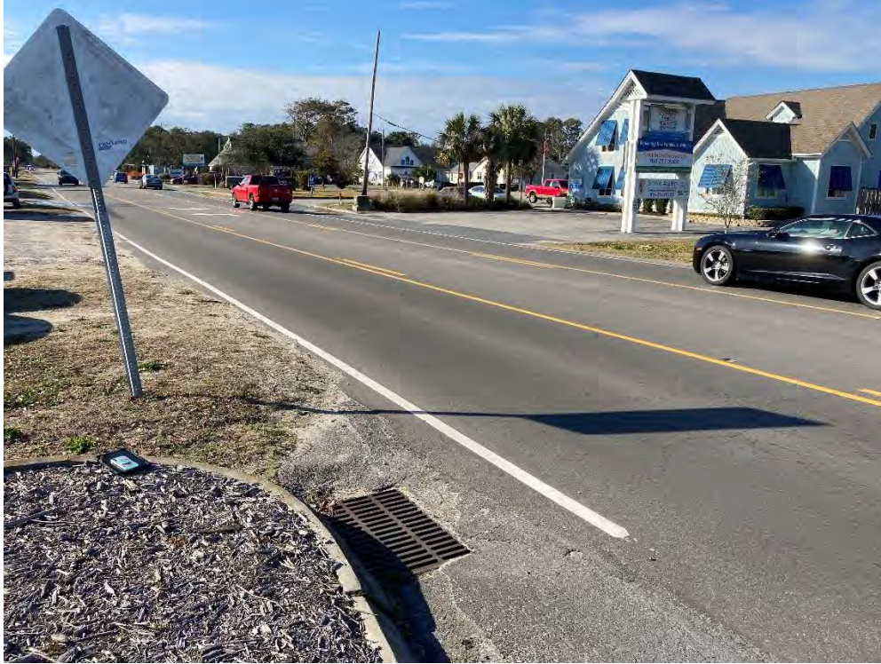
Photo 9: Ex. Inlet @ E. Oak Island Drive and Womble St. View looking North-West.
