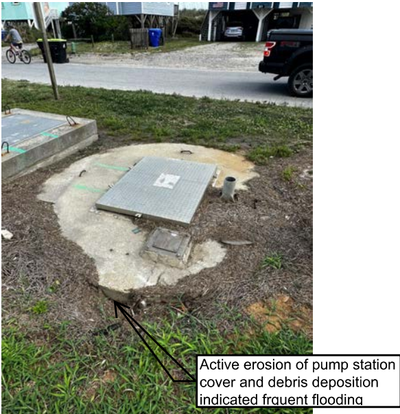
Photo 16: Erosion is occurring around sanitary sewer pump station lid and excess debris indicates frequent inundation.
