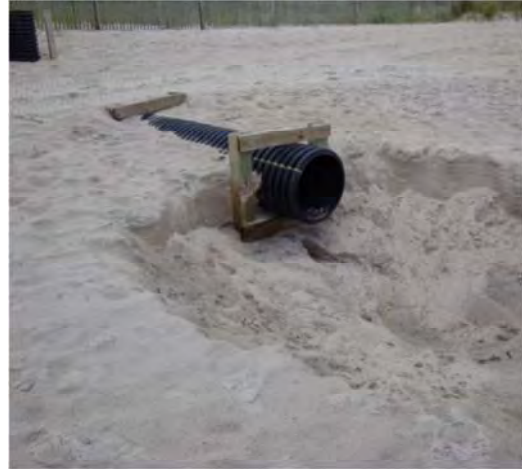
Figure 2. Stormwater discharge pipes are found in many coastal towns in NC. Note the beach scour that is indicative of out flow from a recent storm event.
