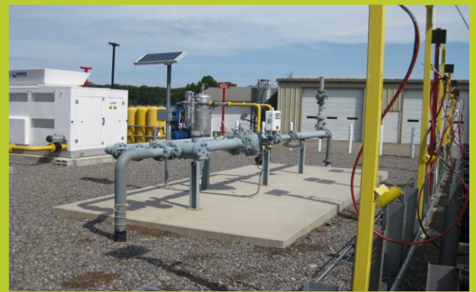
The newly-installed pipe lines that supply compressed natural gas to BSS were gladly received by the local community, who now have access to low-cost CNG as well.
