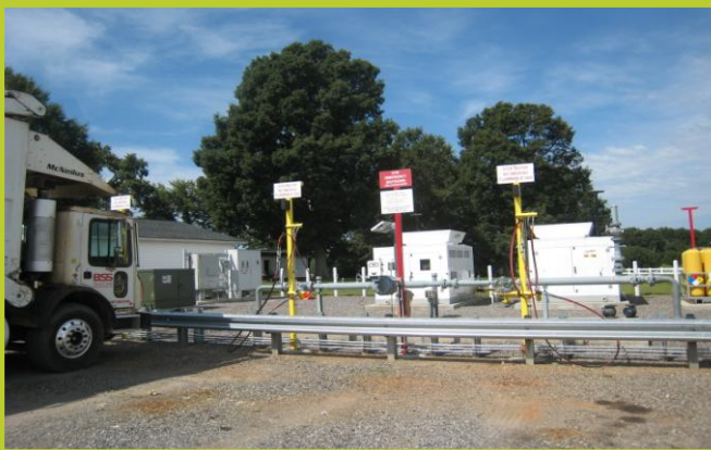
The fill posts were installed to optimize and minimize the space(s) they occupy. Up to 40 posts can be installed on the grounds.
