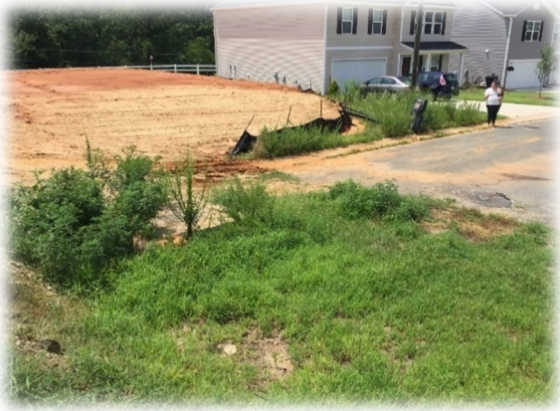
Figure 8 - Poor Practice – No Construction Entrance
