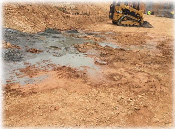
Figure 6 - Unmanaged Concrete Washout
