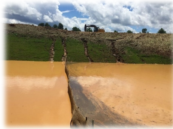
Figure 11 - Rill Erosion on Sediment Basin Slope
