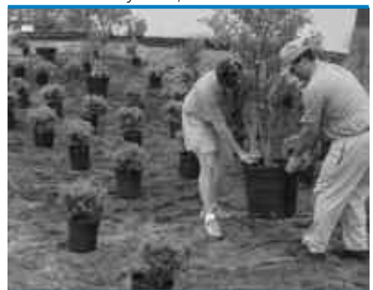
Installation of plants in a rain garden at Carolina Beach State Park Marina.
