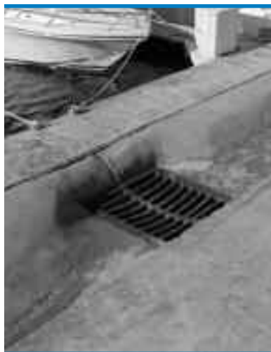
Stormwater inlet draining directly to marina basin.
