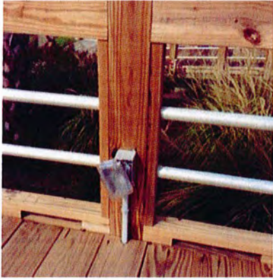
Oct. 3, 2015: Broken electrical outlet cover
