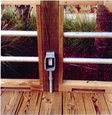
Oct. 3, 2015: Missing cover for electrical outlet
