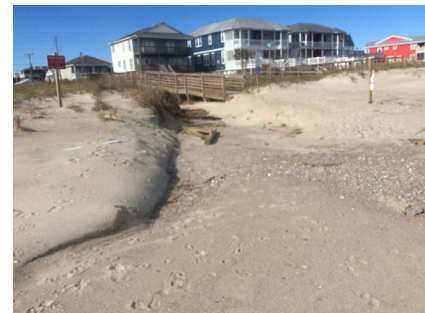
Photo 3: Erosion from overflow area after Hurricane Florence
