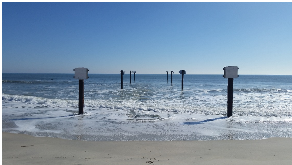
Fig. 3 Outfall buried and extended beyond the surf zone, and marked with warning signs
