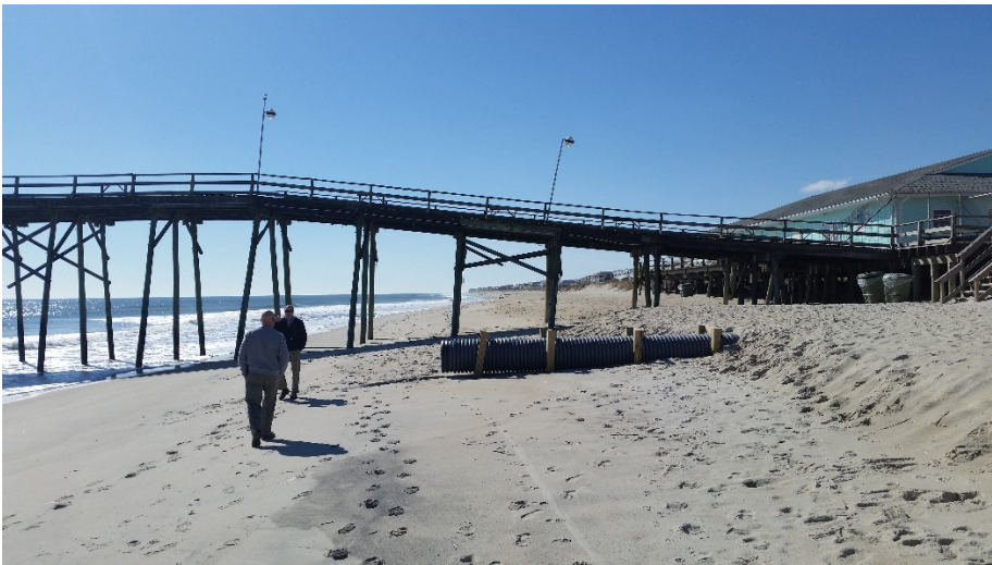
Fig. 2 Exposed outfall pipe and framing on an eroded beach
