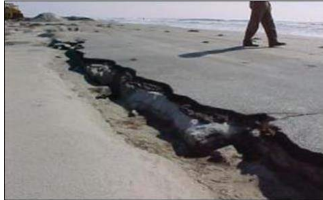
Figure 1. Storm Damaged Section of NC 12
