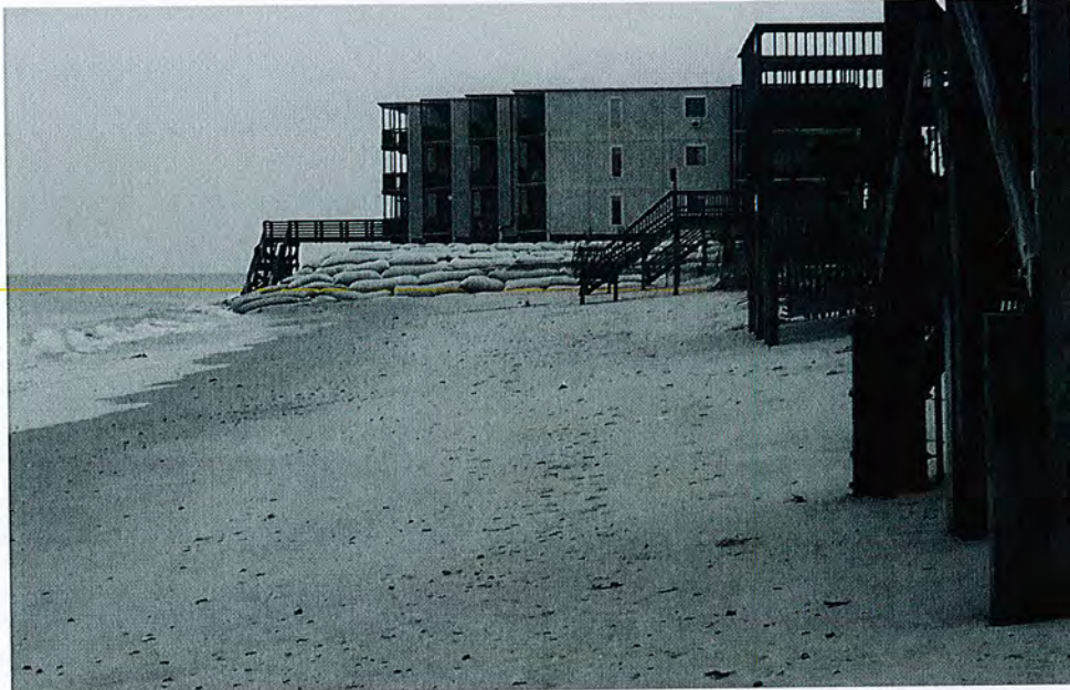
Figure 2. Sandbags revetment at Topsail Reefs Building 1 (Sep 2014).
