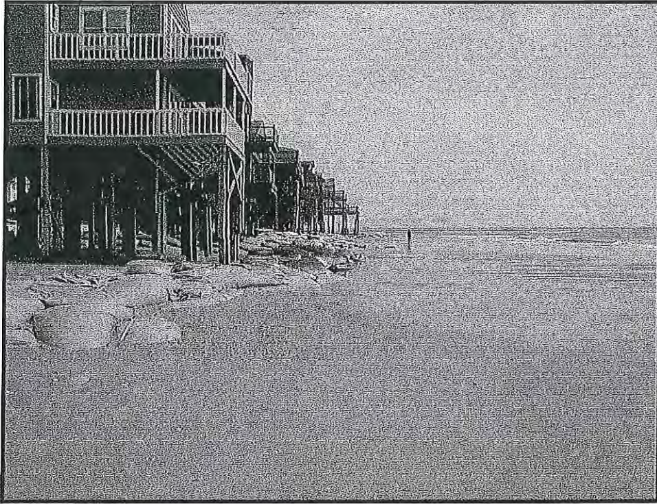
Figure 14. Example of failed sandbag revetment on north end of North Topsail Beach.
