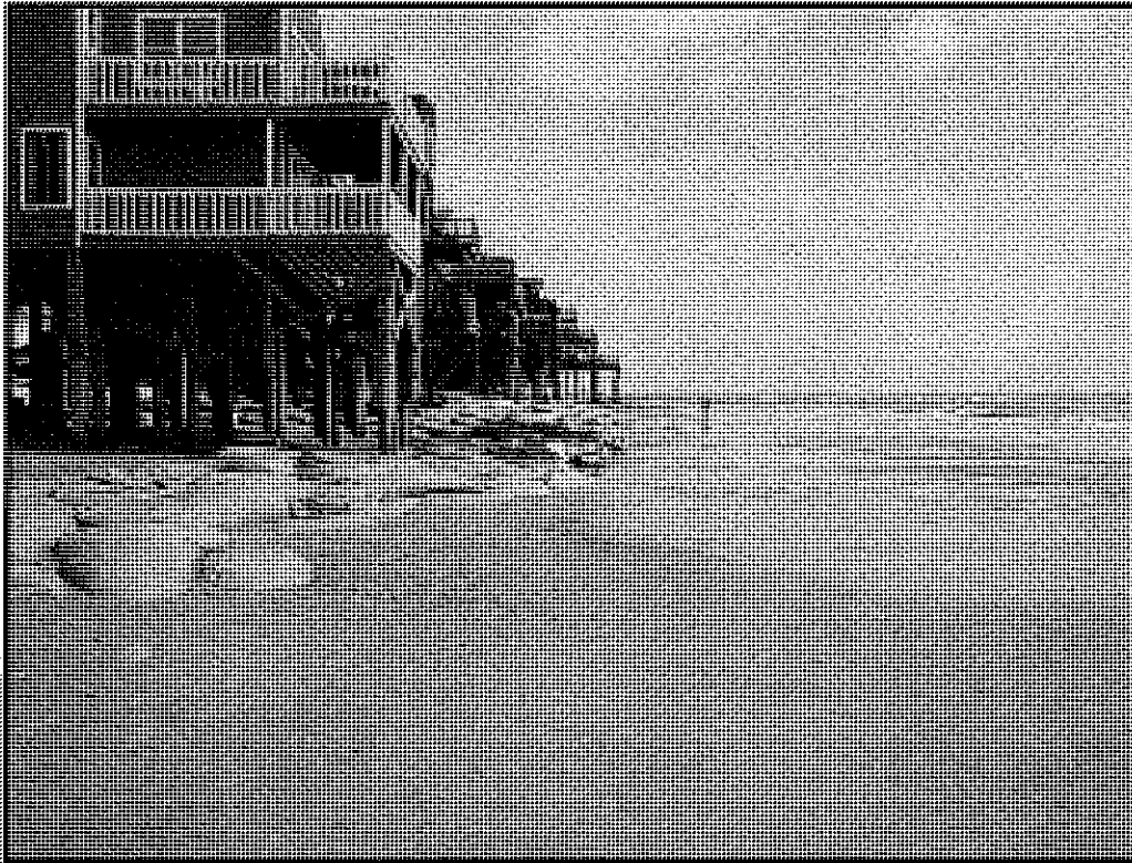
Figure 14. Example of failed sandbag revetment on north end of North Topsail Beach.
