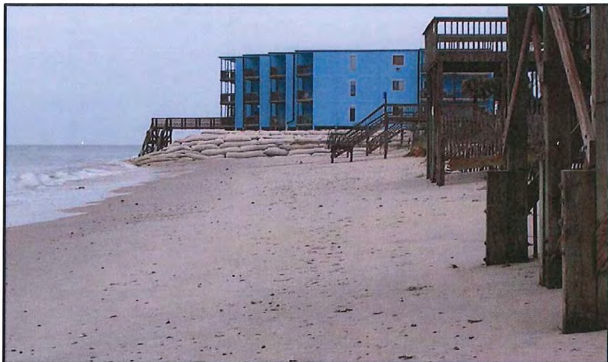
EXHIBIT 8: Sandbags revetment at Topsail Reefs Building 1 (Sep 2014).
