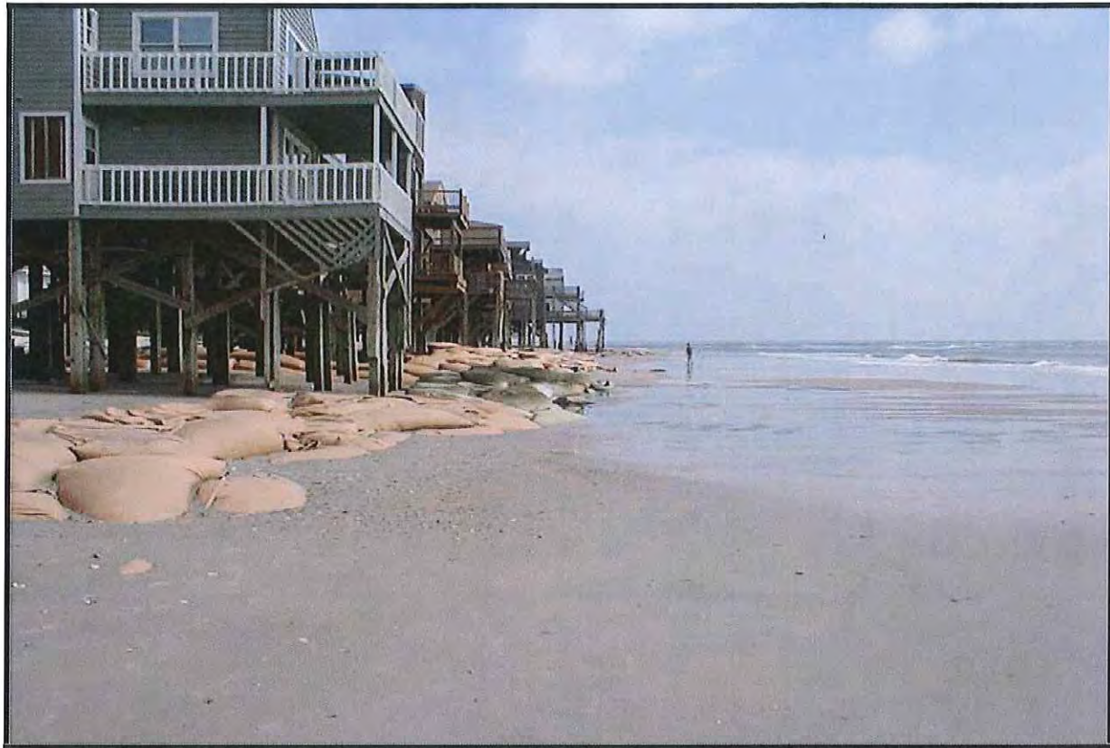
EXHIBIT 7: Example of failed sandbag revetment on north end of North Topsail Beach. Photo taken in September 2005. All of these sandbags and structures, which were located seaward of the present row of homes north of Topsail Reef, have been removed.
