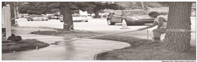
City sidewalks Crews are busy, weather permitting, installing new sidewalks on the west side of North Hesse Street, from St. George Street to 10th Street as part of the "State Routes to Schools" program, partially funded by grant money.
