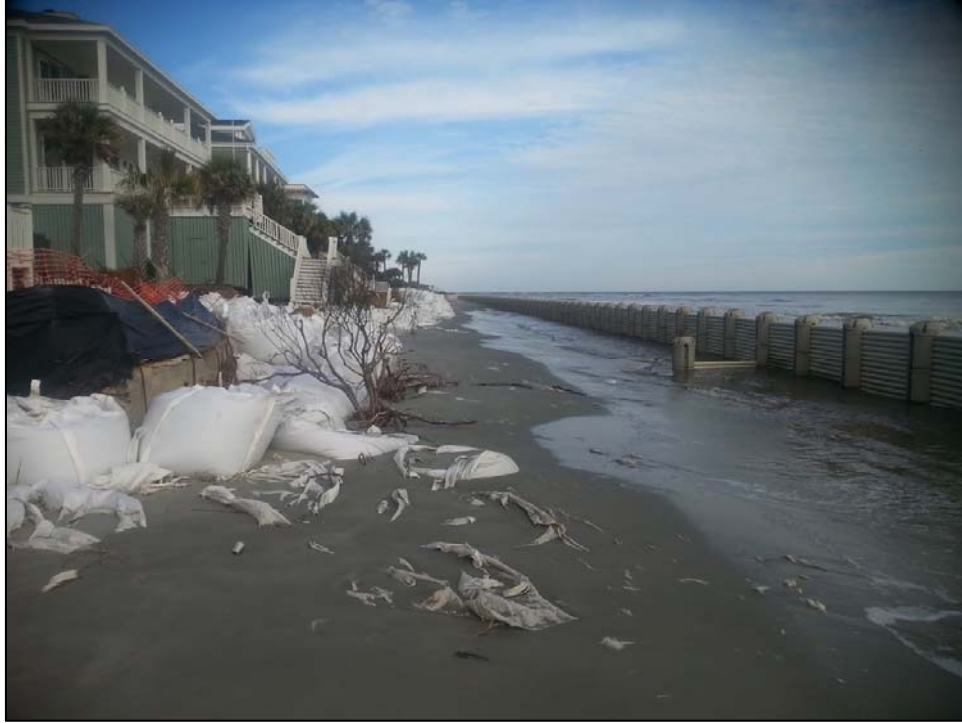
Figure 15. Experimental erosion control structure installed at land-ocean interface at Isle of Palms, S.C. with partially damaged sandbags behind the structure. Photo: NCDCEM, 2015
