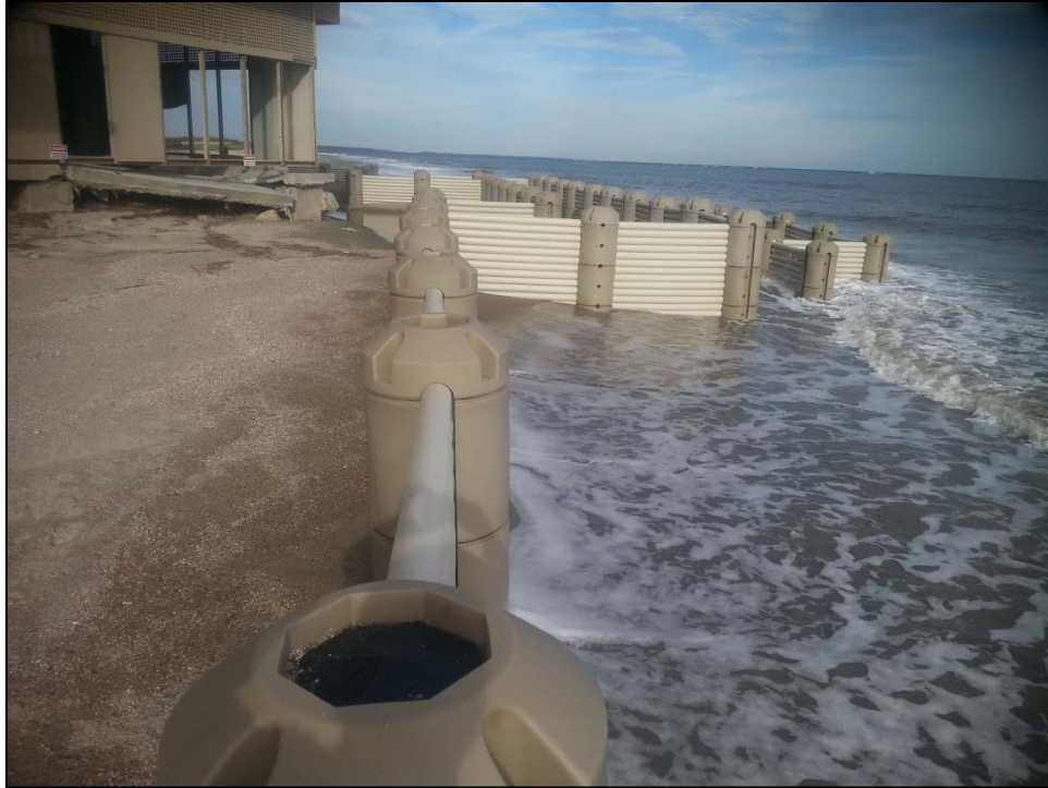
Figure 17. Experimental structure at Isle of Palms, S.C., where sediment appears to have been retained on the landward side of the structure, while the dry sand beach on the ocean side appears to have been lost to erosion. Photo: NCDCCM, 2015
