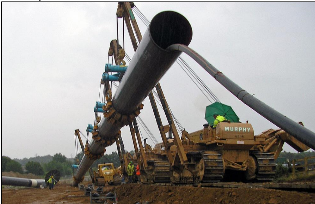
FIGURE VII(f) – Final section of pullback pipe for an HDD operation in relatively flat terrain.
