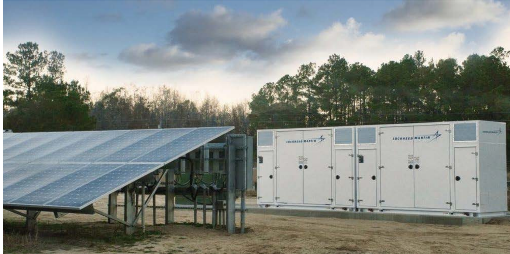
Brunswick EMC and Cypress Creek's 12 MWh Solar+Storage Project
