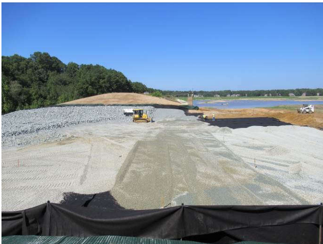
Upstream breach covered by bedding stone and graded
