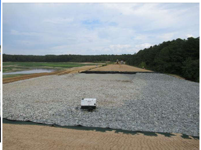
The majority of the breach is armored with riprap
