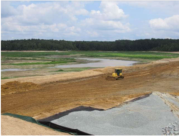
The upstream area of the breach is graded in preparation for placement of fabric
