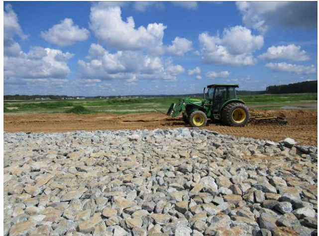
The upstream area of the breach and cofferdam are tilled prior to seeding
