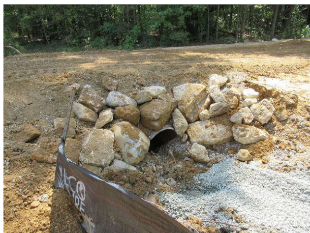
Reinstallation of the water diversion pipe at the entrance to the staging area
