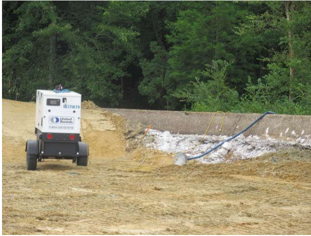
The pump for dewatering the spillway
