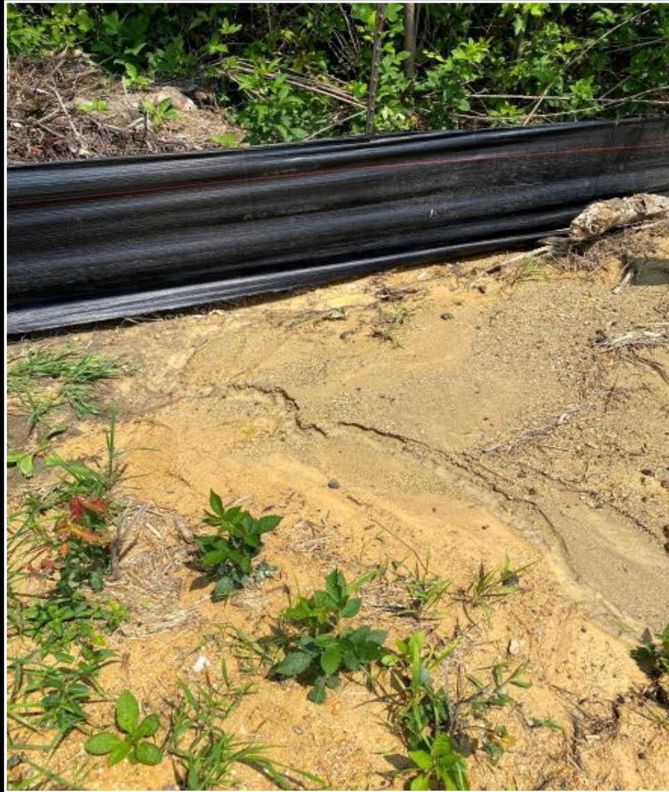
Undercut and unsecured silt fence
