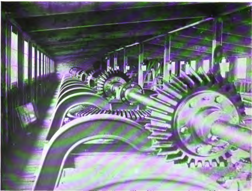
B.—INTERIOR VIEW, UPPER PART OF POWER-HOUSE, FRIES MANUFACTURING AND POWER CO.
