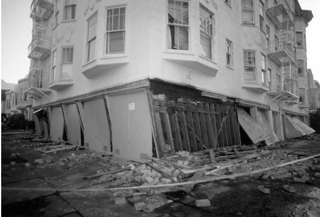
Figure 5. “Soft” or weak first story failure of a four-story building in San Francisco damaged by the October, 1989 Loma Prieta earthquake. In this case the weak story is caused by reduced shear wall strength and lack of diagonal bracing related to constructing parking garages (note garage doors) in the first story of the building.
