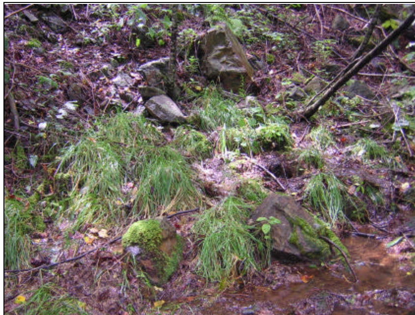
Figure 10. Seepage (~10 gallons per minute) from base of man-made rock slope (bottom right of photo) at Site 3. Downslope is toward bottom right.
