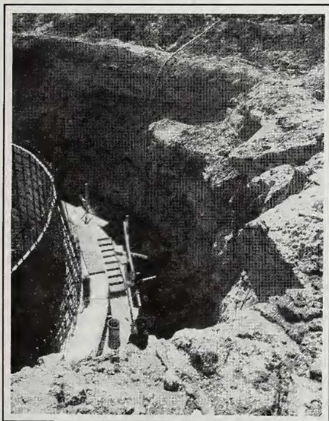
Figure 10. Exposure of Trcs facies in sewer excavation east of Page Road (SR 1973) at Interstate 40 (Locality 14).
