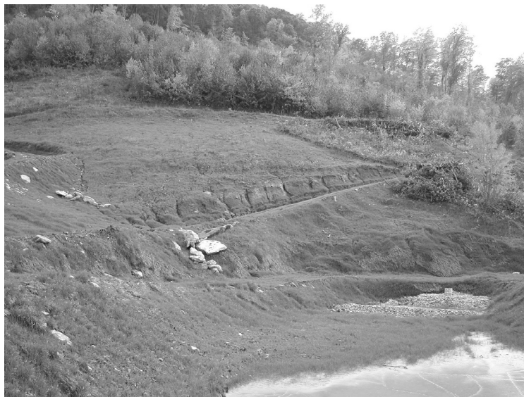
First basin completed at Sports Garden and the site stabilized with grass.
