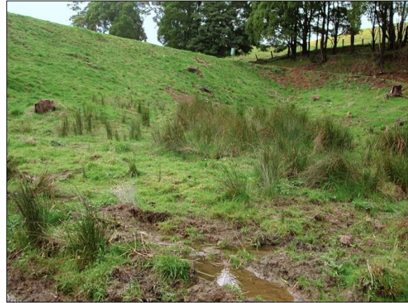
Earthen dam seepage
