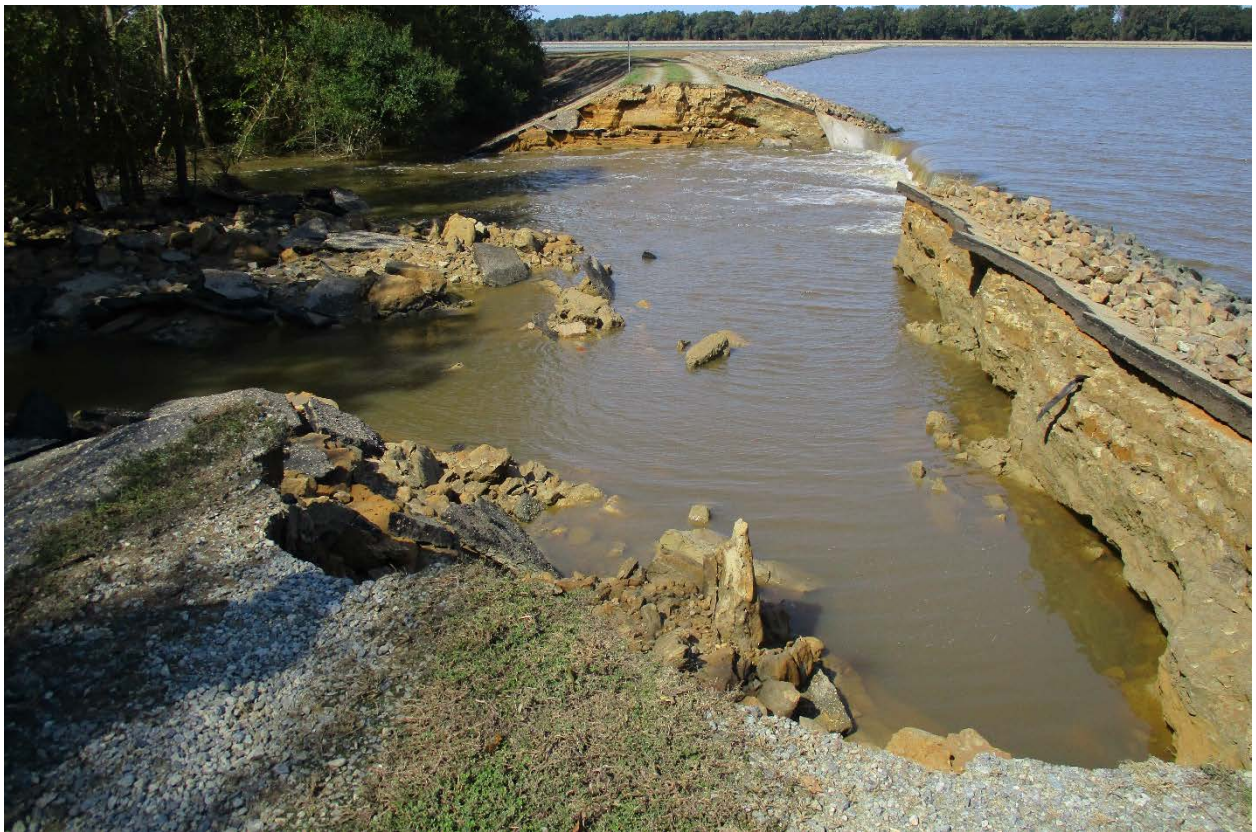
Figure 8.8 H.F. Lee Cooling Pond Partial Breach; Credit: NC DEMLR
