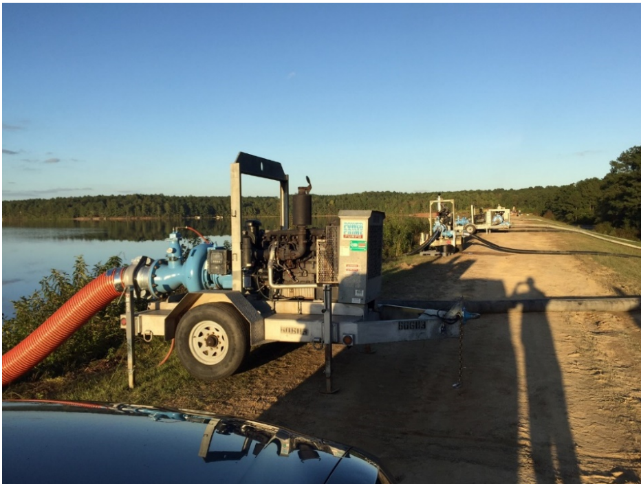
Figure 8.2 Pumps on Woodlake Dam Crest;
