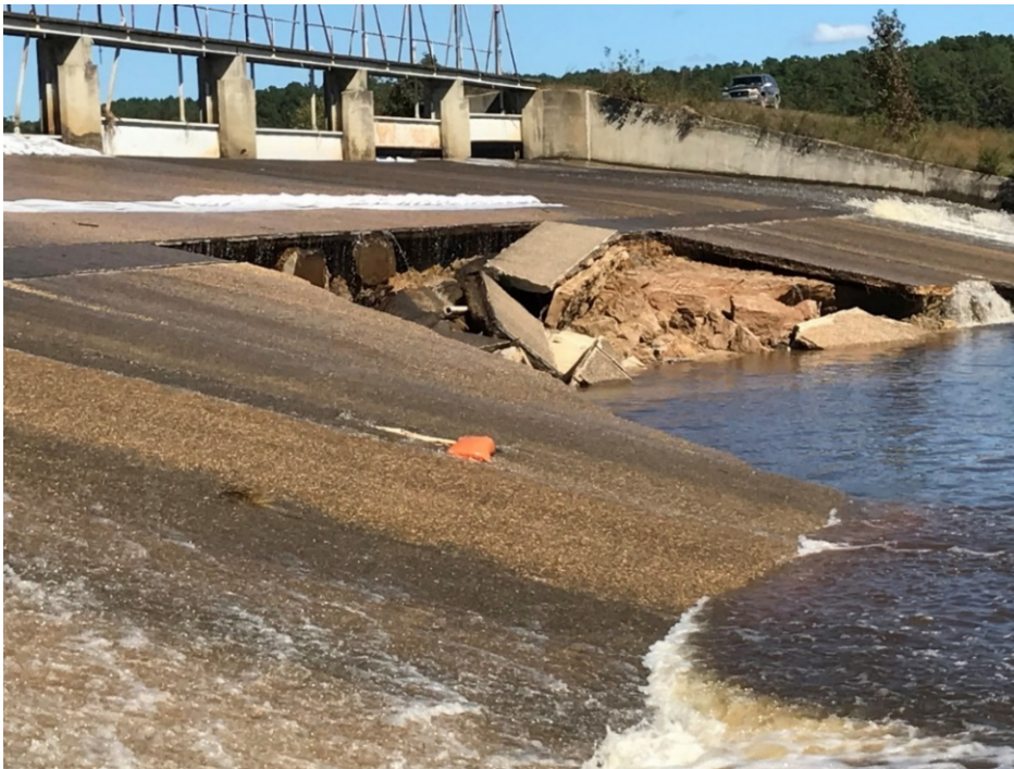
Figure 8.1 Damaged concrete spillway at Woodlake Dam Credit: NC DEMLR
