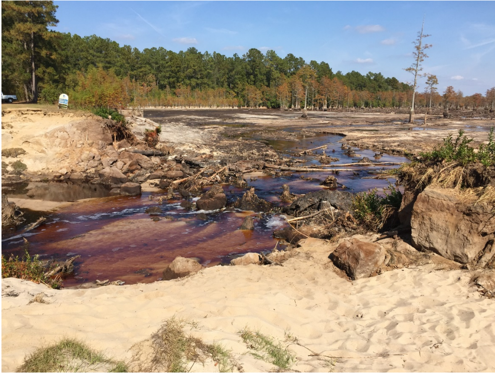
Figure 11.2 Jessup Mill Pond breach (Smith Lake Dam); Credit: FEMA; Plisich
