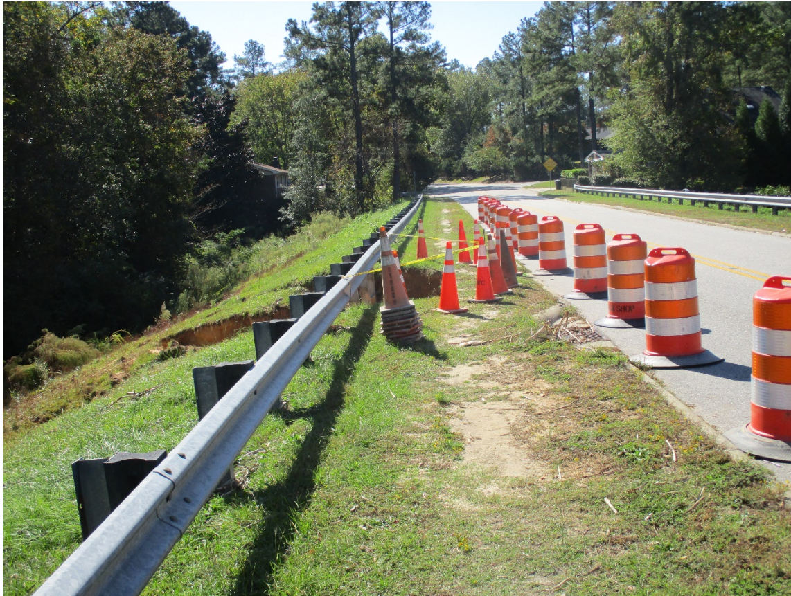
Figure A9.4: Devonwood Lower Dam post-event photo;
