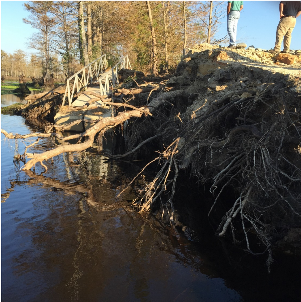
Figure A5.5: Rhodes Lake Dam root system in failed dam embankment left of spillway; same root system seen in Fig A5.4; October 31, 2016 Credit: FEMA; Plisich
