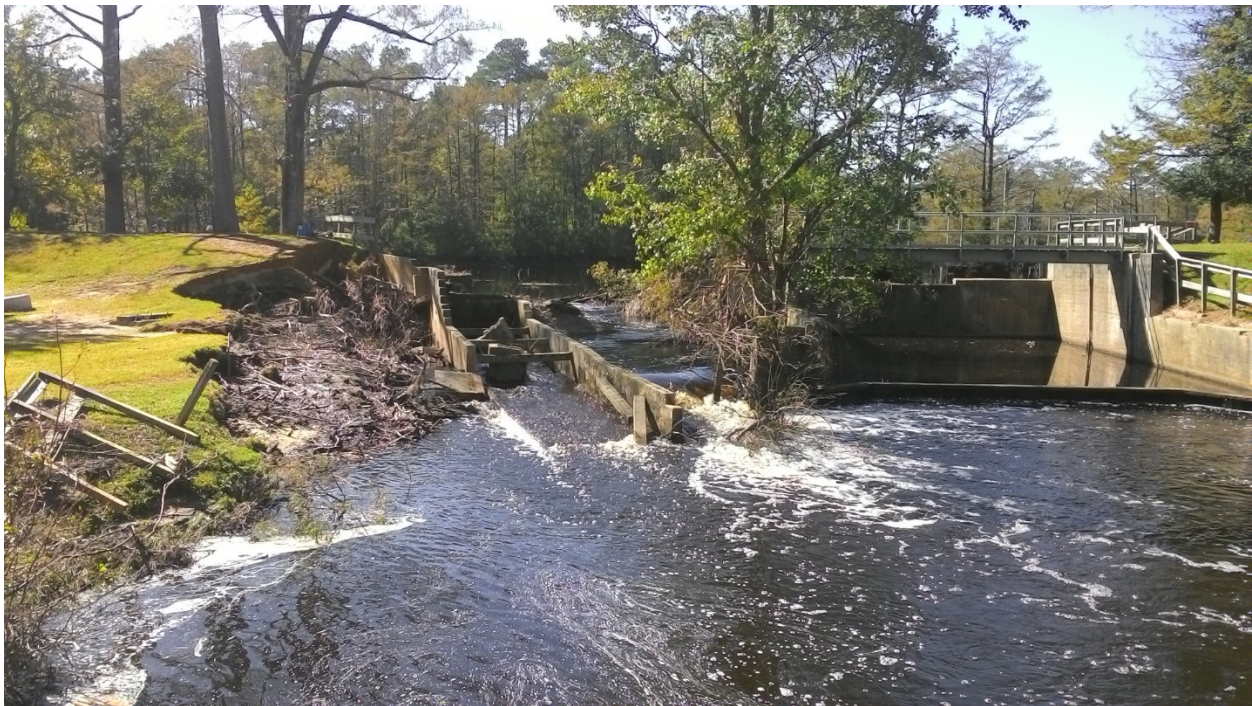
Figure A15.5: Tull Mill Pond Dam post-event photo; Note trees on embankment and tree root system within embankment Credit: NC DEMLR
