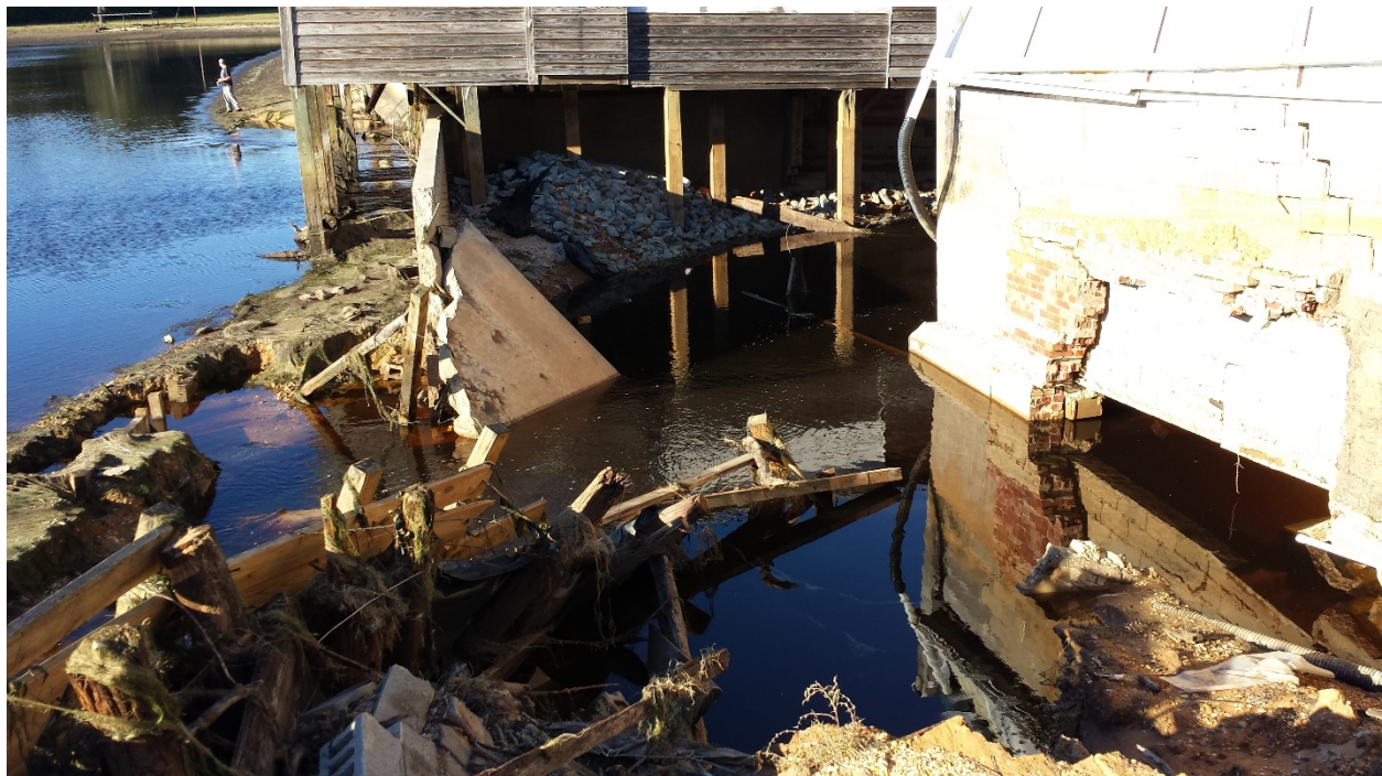
Figure A17.4: House Autry Dam post-event photo;
