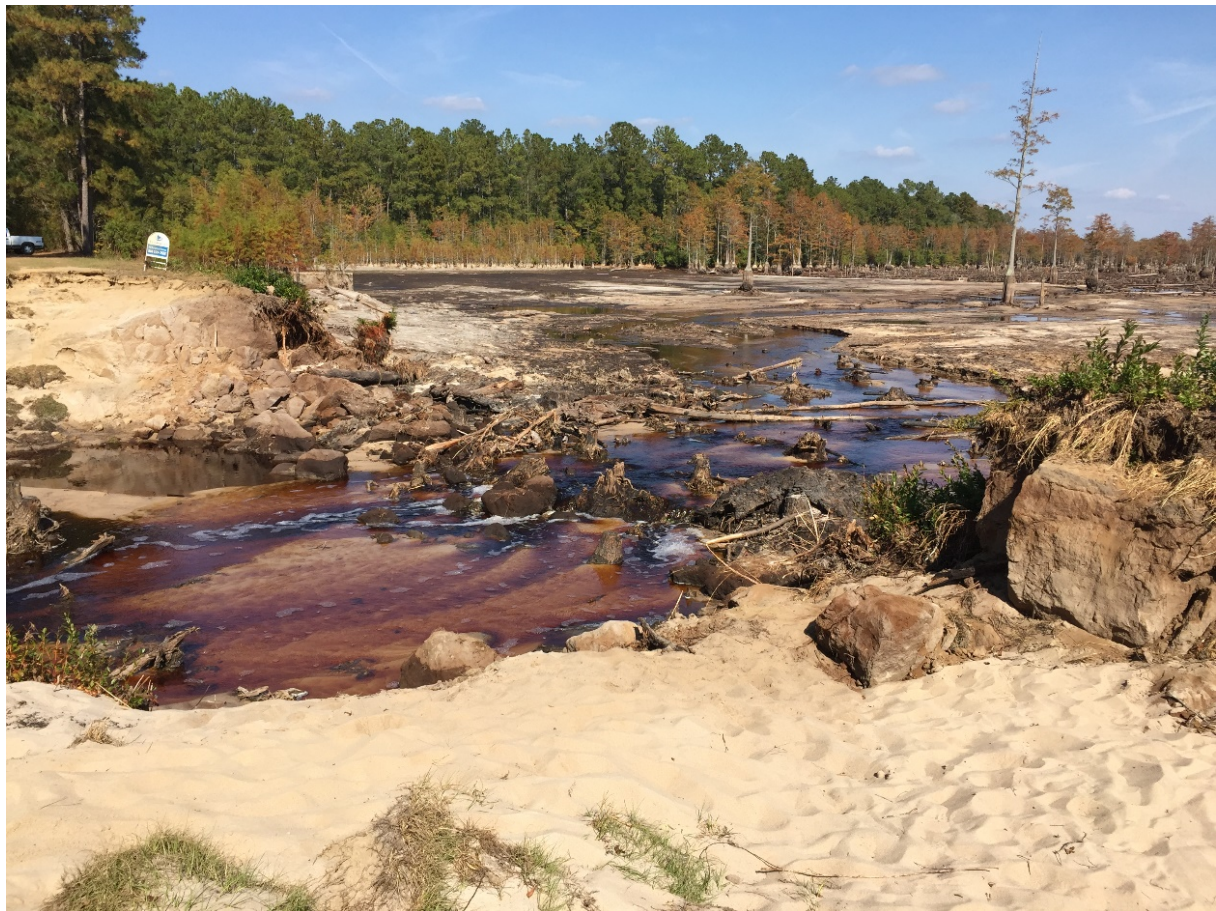
Figure A3.4: Smith Lake Dam post-event photo; Credit:
