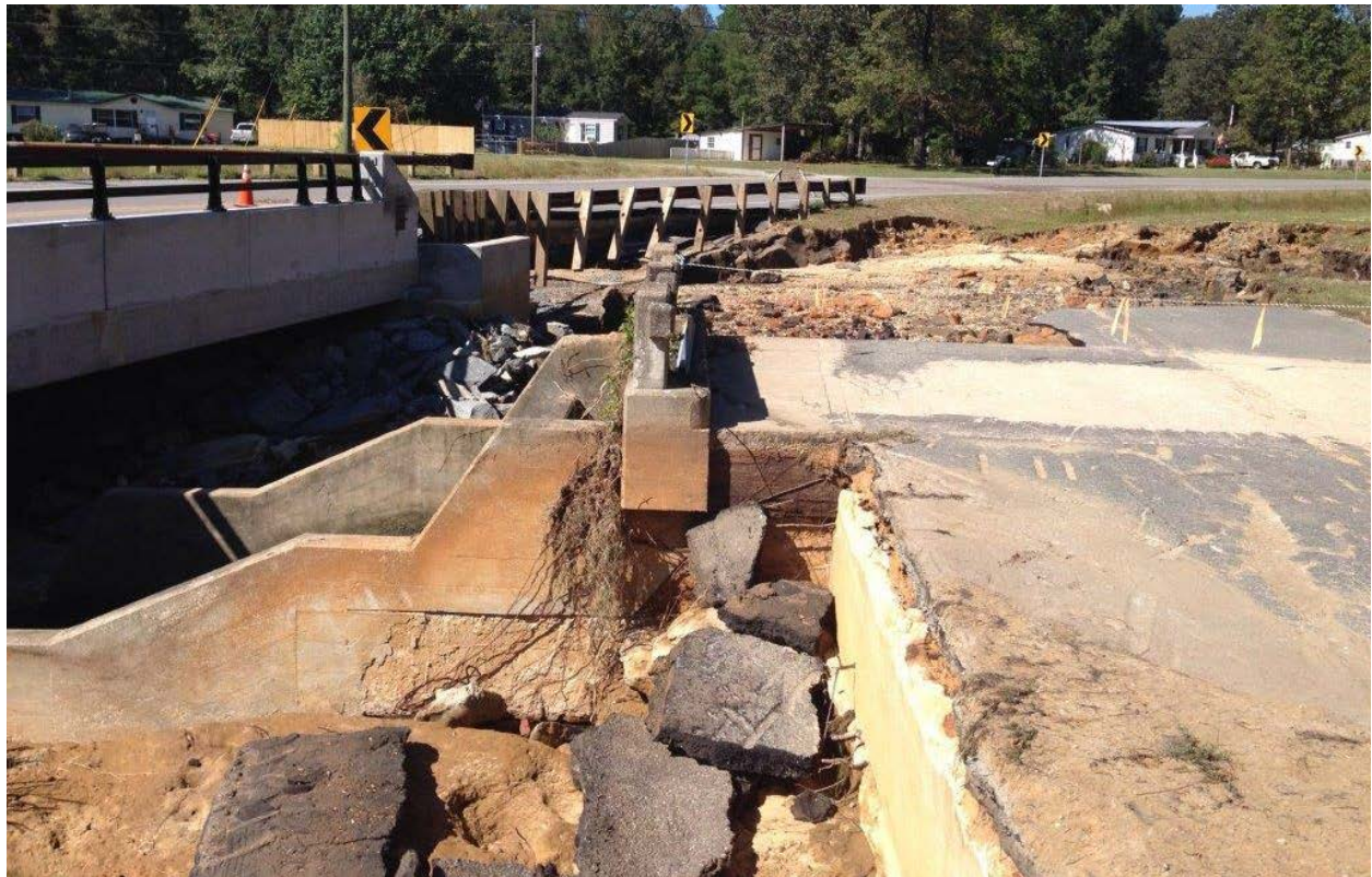
Figure A12.5: Maxwell Mill Pond Dam post-event photo;
