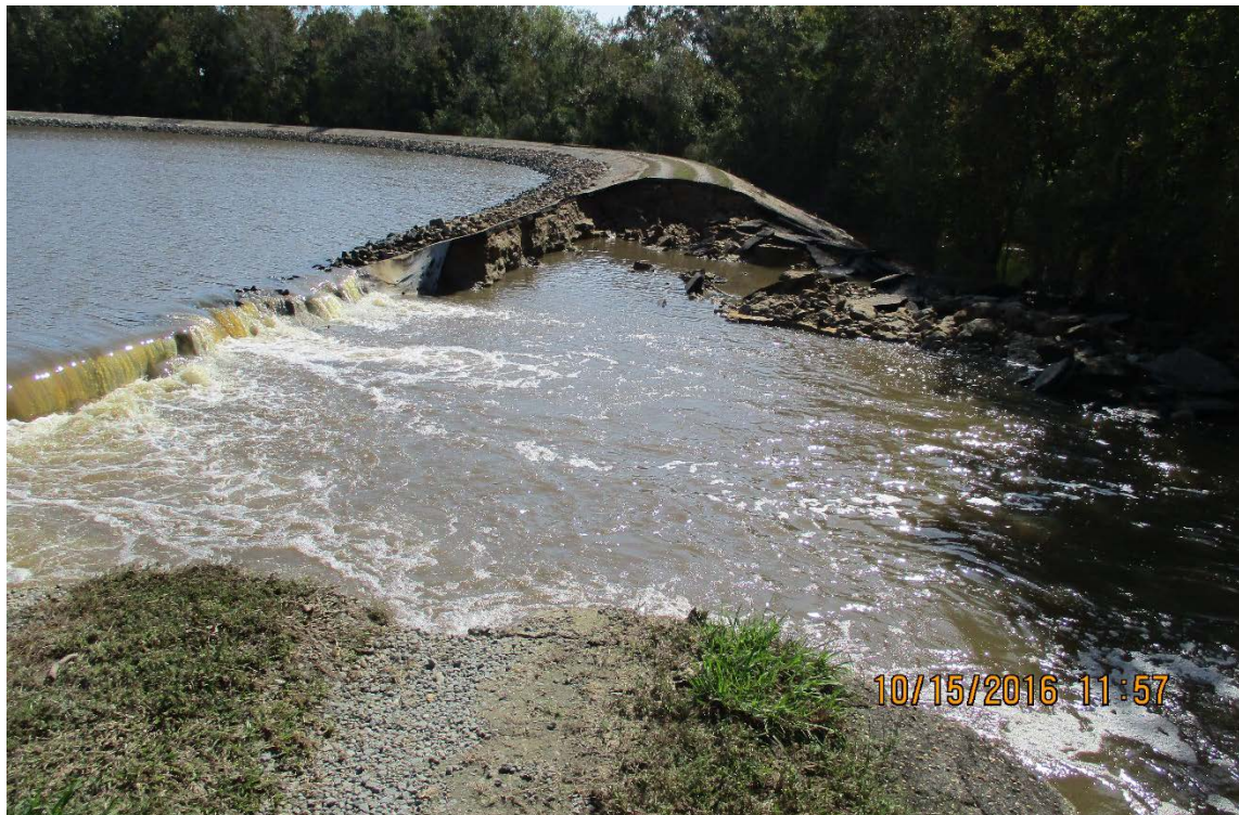
Figure A19.5: H.F. Lee Power Station Cooling Lake Dam post-event photo; Credit: NC DEMLR
