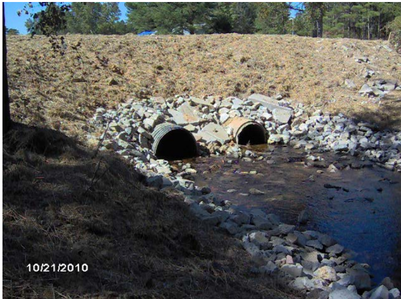
Figure A14.1: Former Sunset Lake Dam turned into dry retention pond; pre-event image; October 21, 2010 Credit: NC DEML
