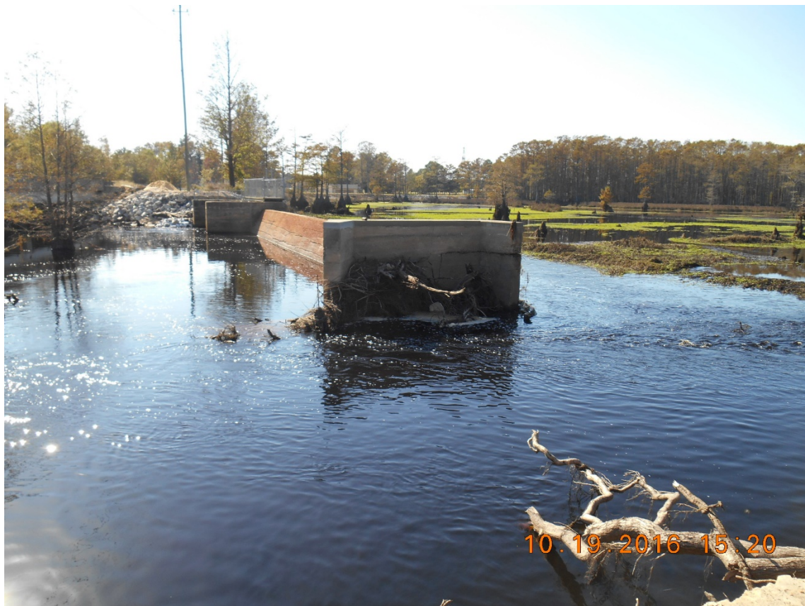
Figure A5.4: Rhodes Lake Dam failed left embankment nearest the spillway post-event photo; Note the root system in foreground in the embankment; October 19, 2016; Credit: NC DEMLR
