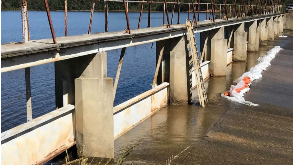
Figure 8.4 Sandbags in center above damaged spillway area; Credit: NC DEMLR
