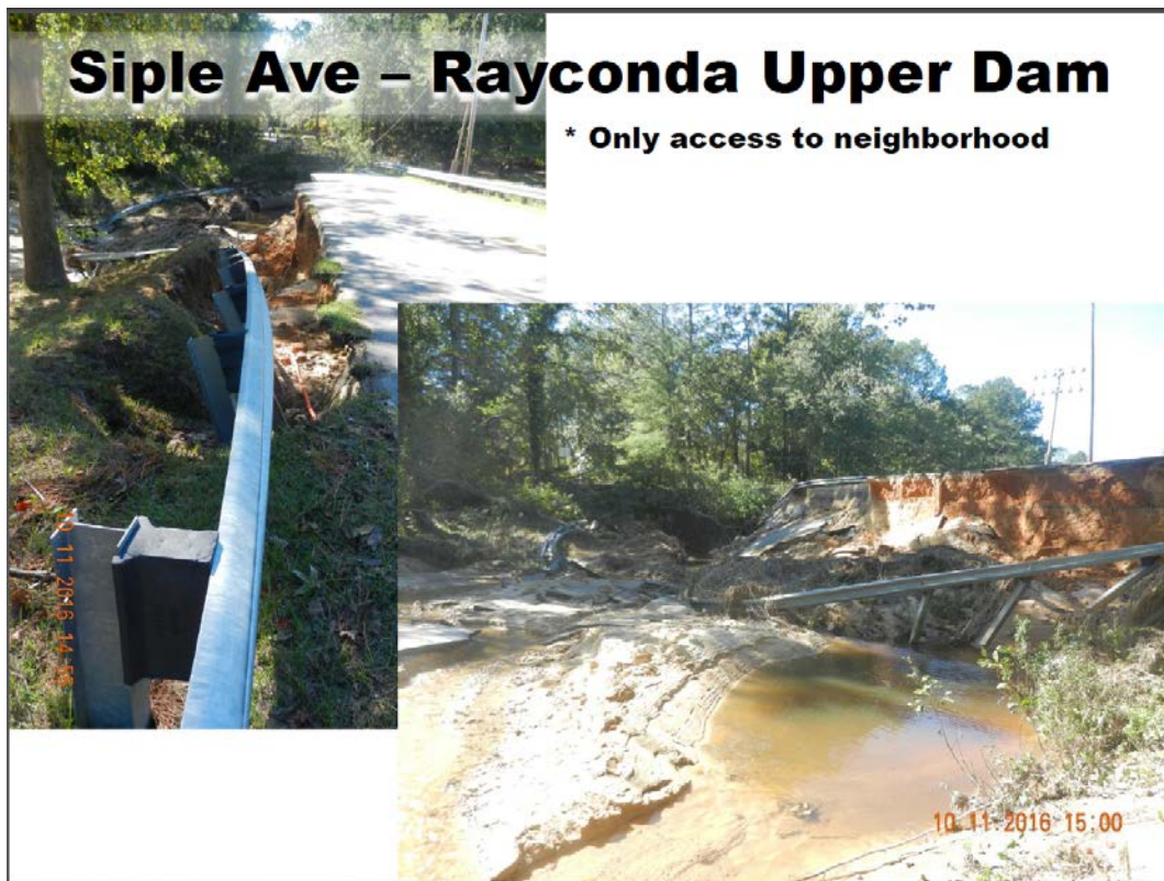
Figure A10.4: Rayconda Upper Dam post-event photo; Credit: NC DEMLR
