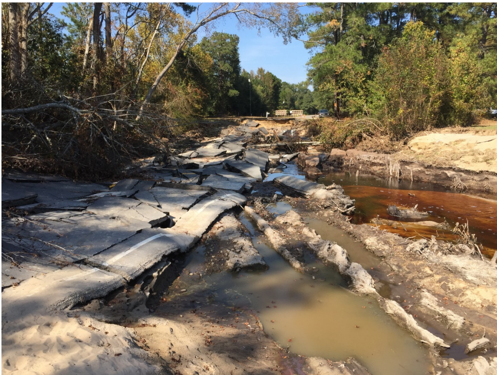
Figure 11.3 State route (NC-53) road washout due to Jessup Mill Pond (Smith Lake Dam) breach; Credit: FEMA; Plisich
