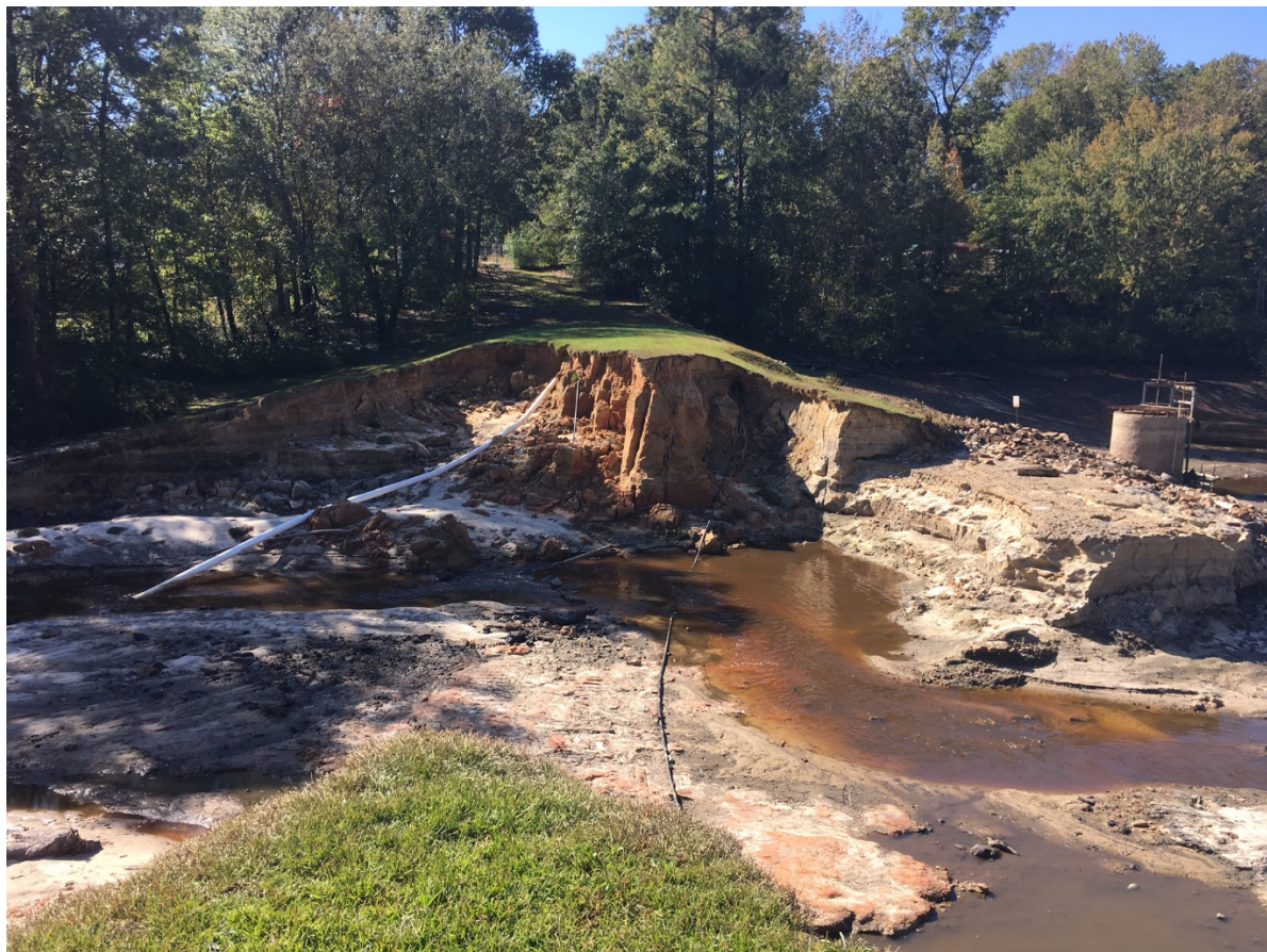
Figure A1.4: Loch Lommond Dam post-event photo;
