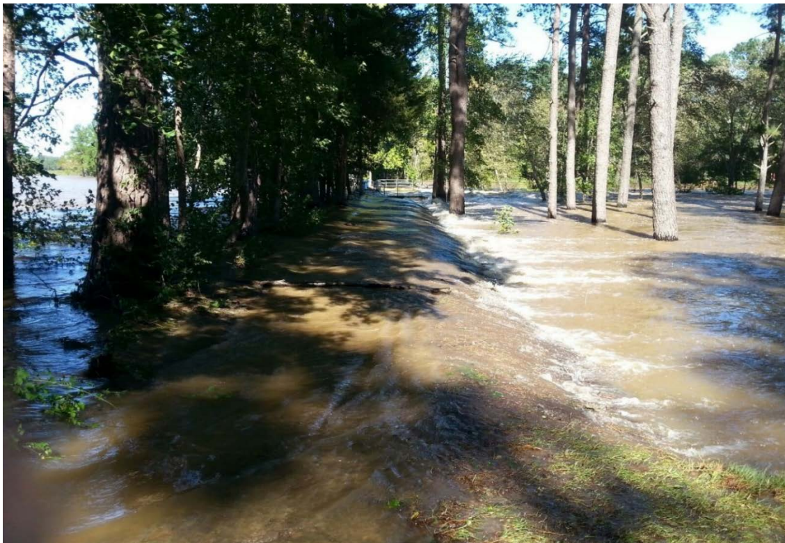
Figure 8.11 Lake Wilson Dam overtopping
