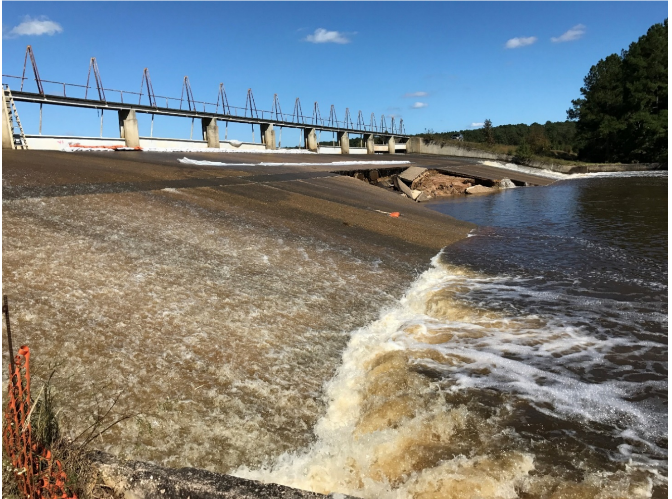
Woodlake Dam (Moore County) post-flooding event;
