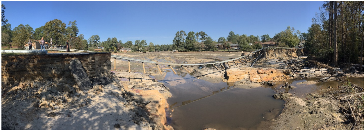
Figure A4.5: Arran Lake Dam post-event photo; Credit: NC DEMLR
