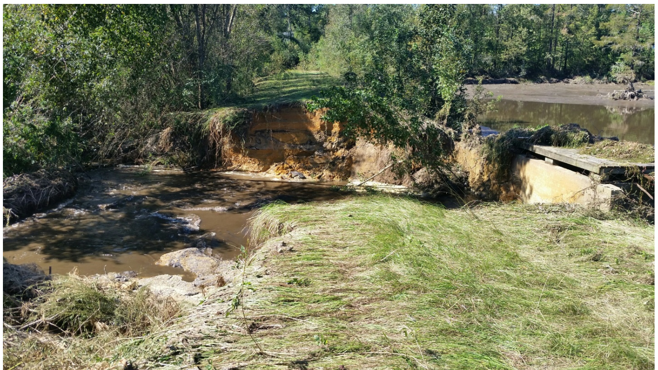
Figure A16.4: Laurel Lake Dam post-event photo;
