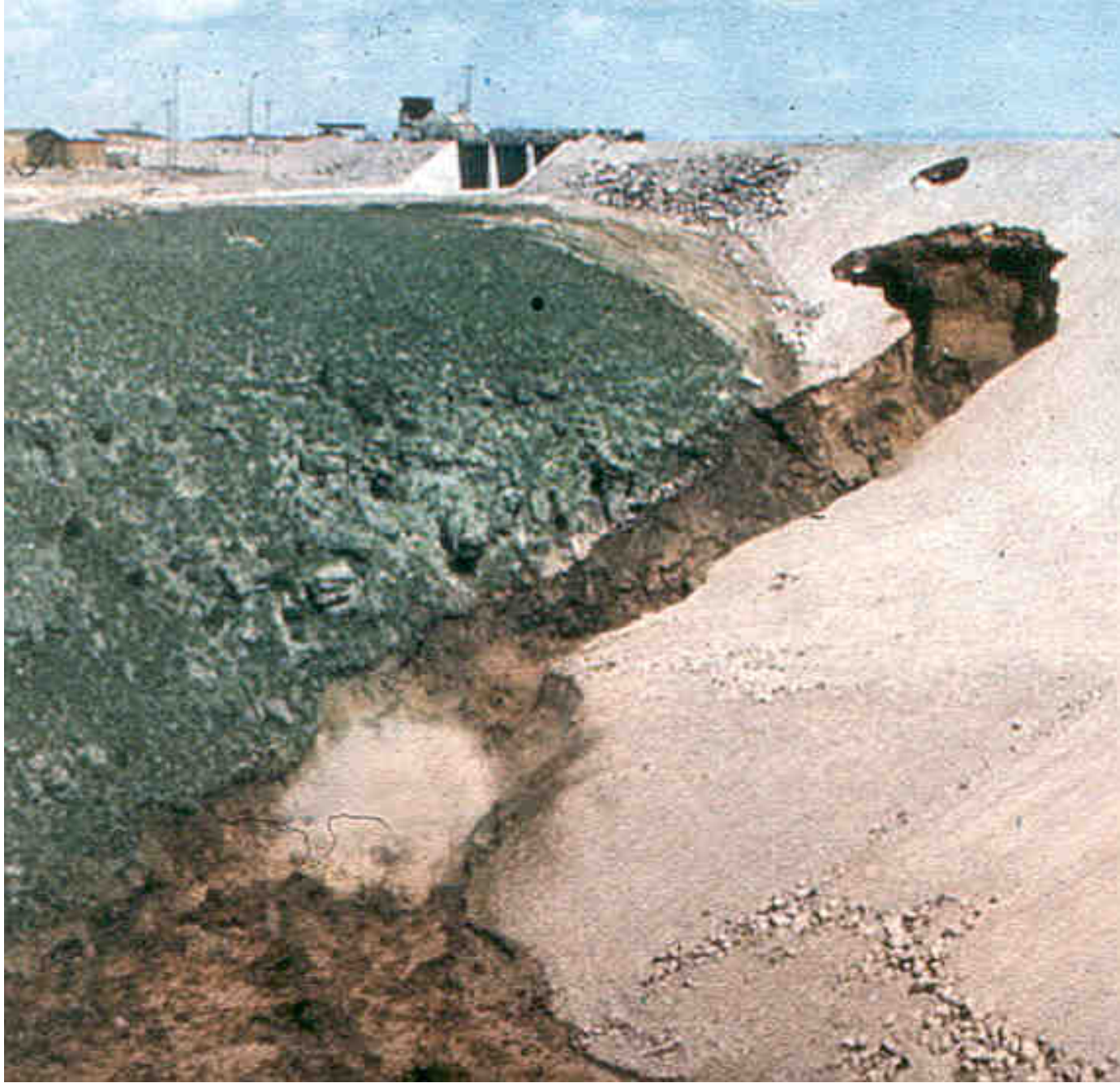
Second Hole in Dam about 11:32 am, June 5, 1976
