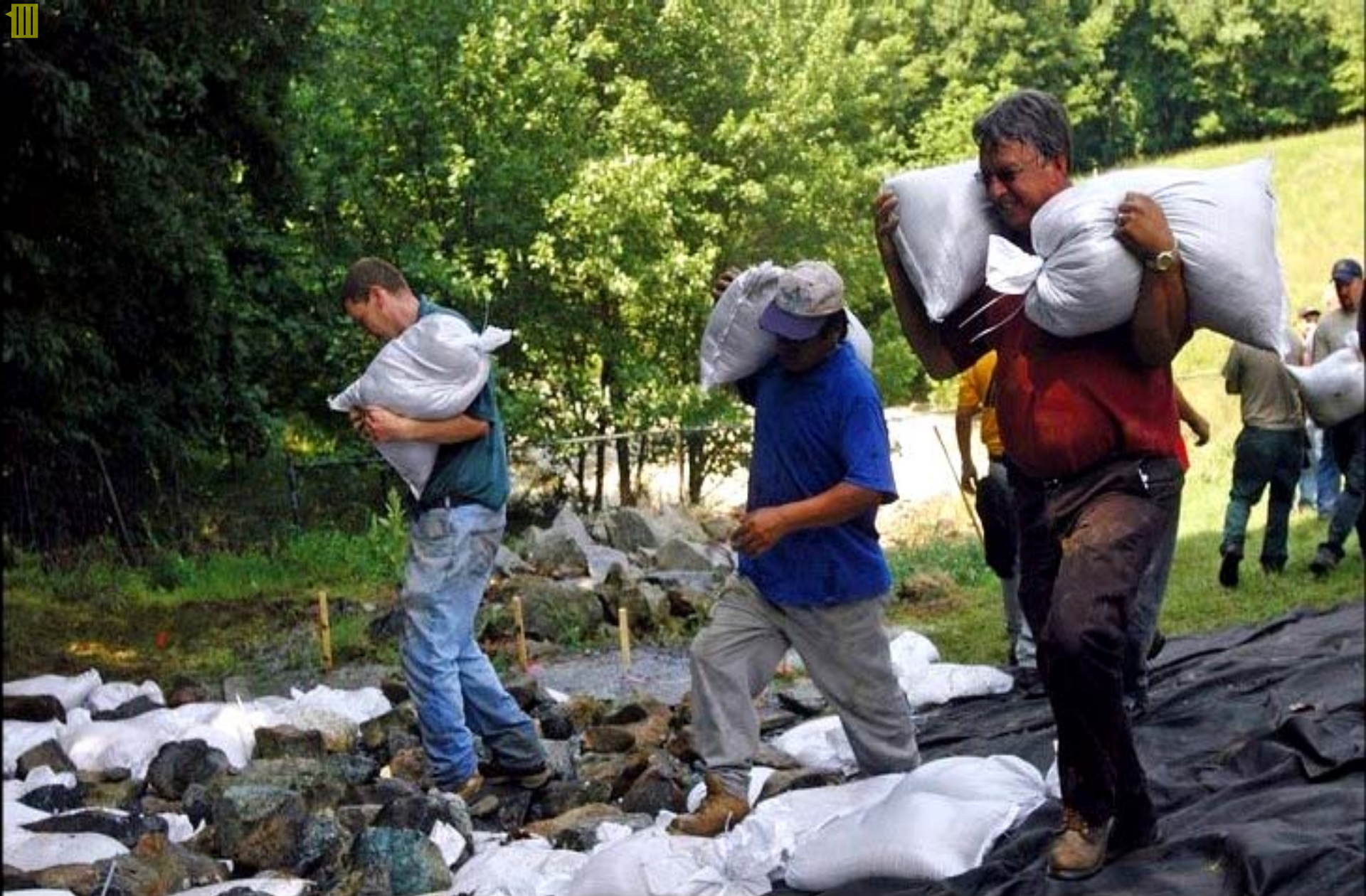
Area workers use sandbags as a temporary fix to stop the over flooding at the dam. Engineers and workers repair the damaged dam at Lake Needwood in Rock Creek Regional Park. The lake is 25 feet about normal and over 2,300 local residents were forced to evacuate.
