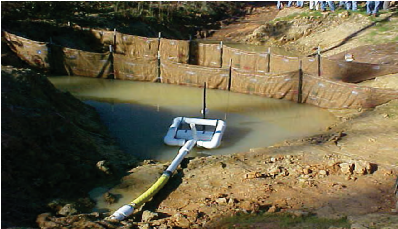
Skimmer sediment basins dewater the sedimentation pool from the surface to ensure the highest quality water is being discharged.
