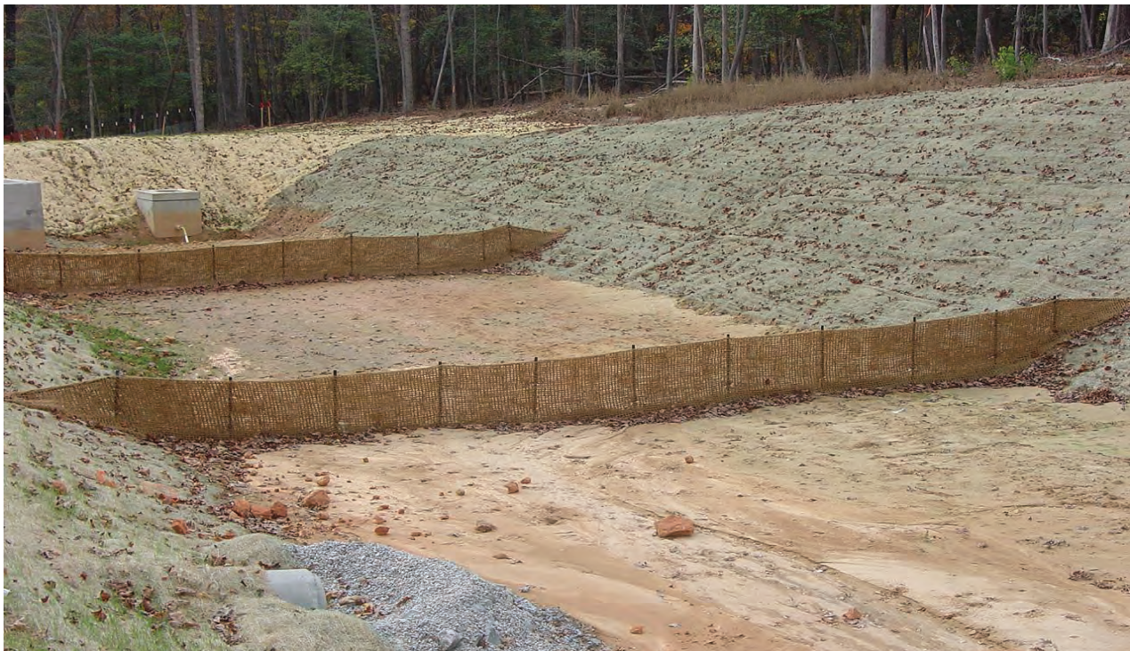
Baffles reduces the velocity and turbulence of water flowing through a measure and assists in the settling of sediment before the water exits the site.
