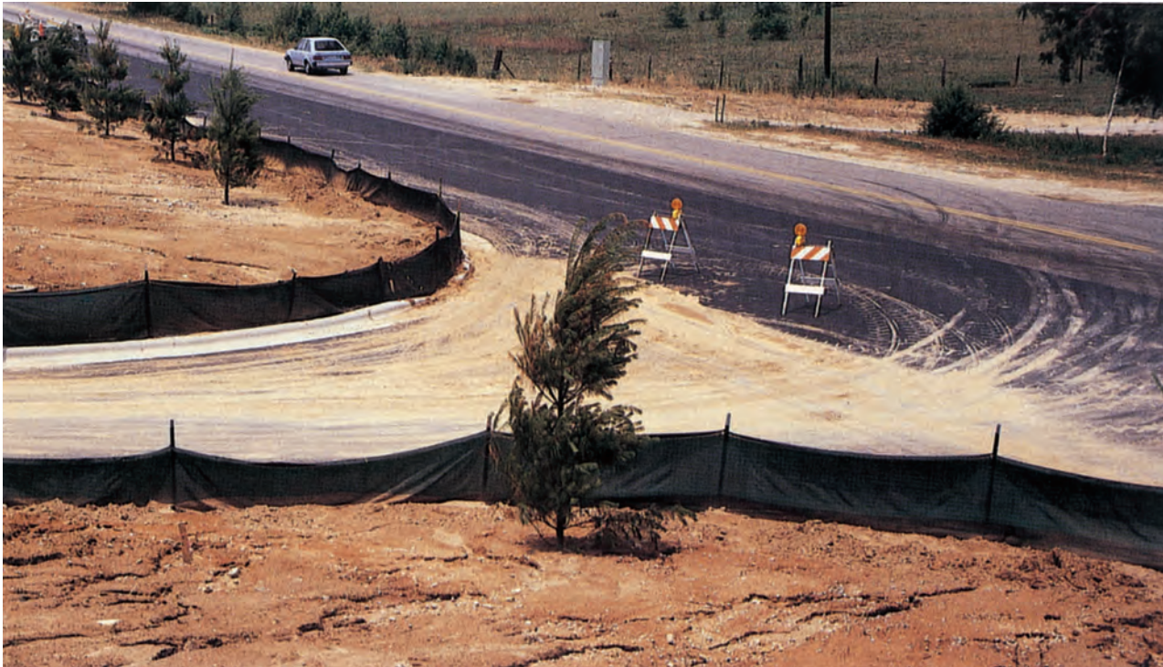
Sediment fences help prevent off-site sedimentation when properly located, installed, and maintained.
