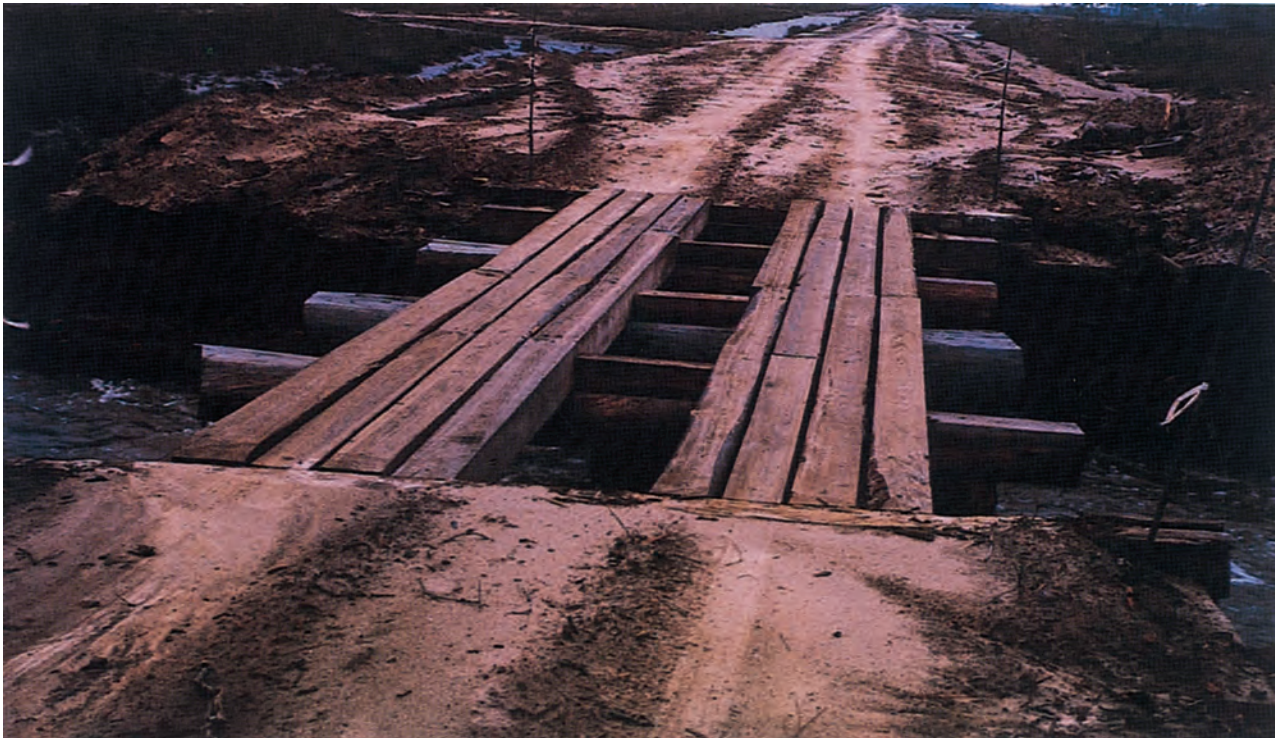
Temporary stream crossing may be a ford, culvert or bridge. Bridges allow full stream flow, but must be designed and built to support expected loads.
