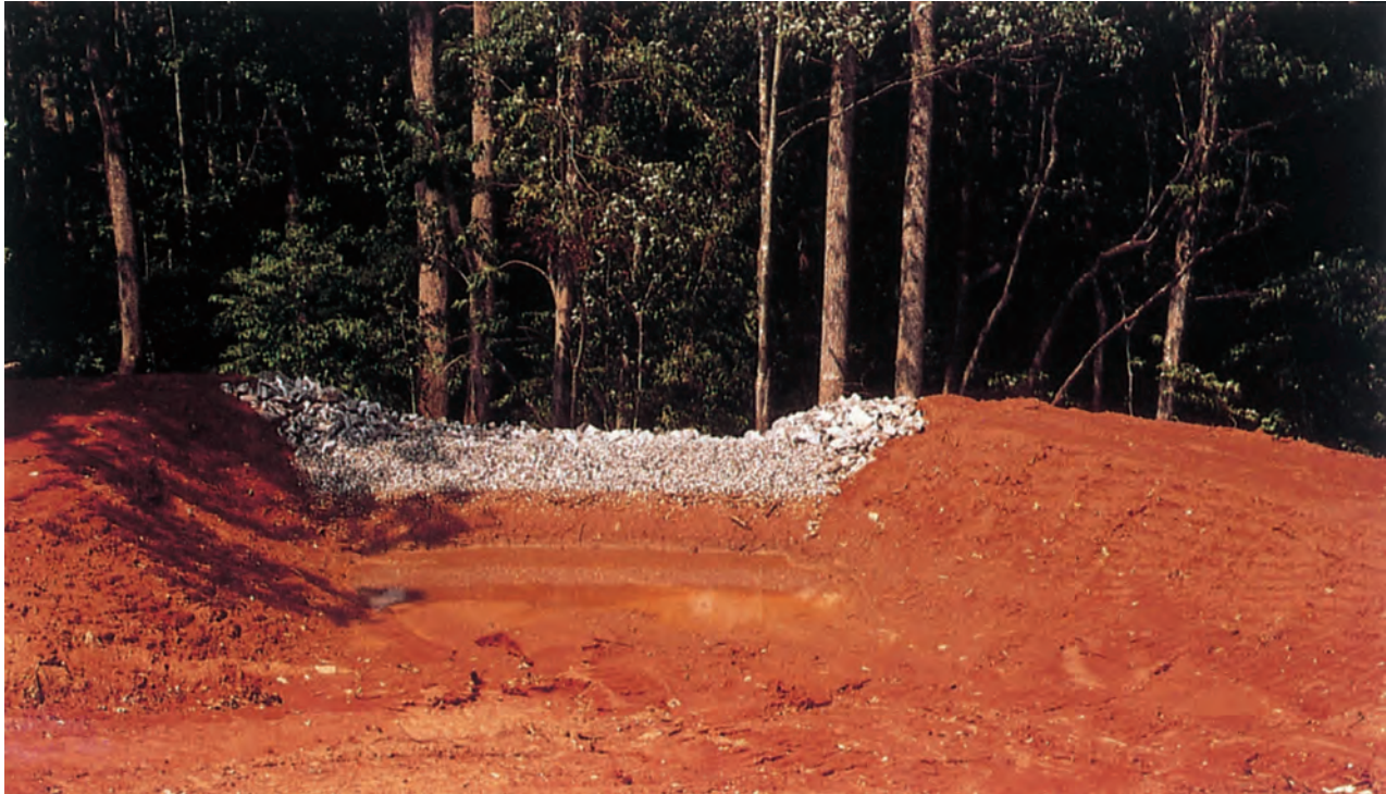
Temporary sediment trap provides a settling pool for a small drainage area. Gravel allows dewatering and a stable outlet.
