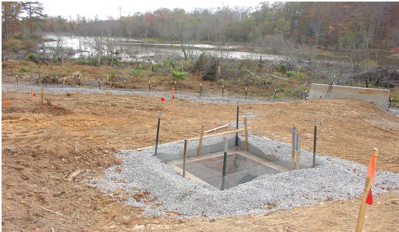
Hardware cloth and gravel inlet protection keeps sediment and debris from construction out of this drop inlet.
