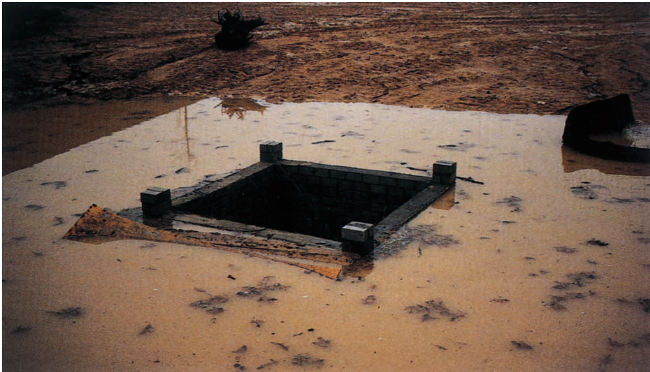
Temporary excavated drop inlet protection creates an effective settling pool to remove sediment at a stormwater inlet.
