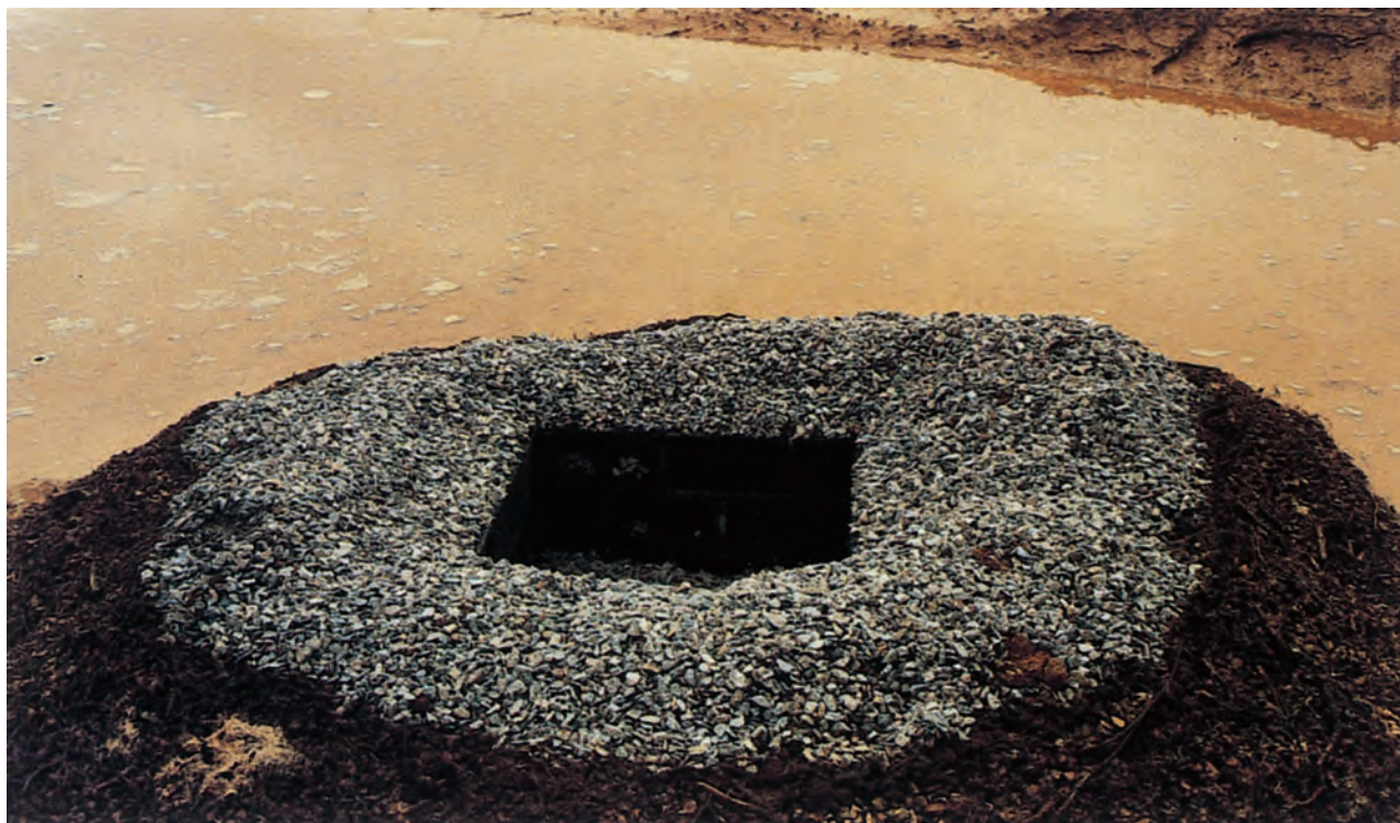
Block and gravel inlet protection prevents sediment from entering this storm drain during construction.
