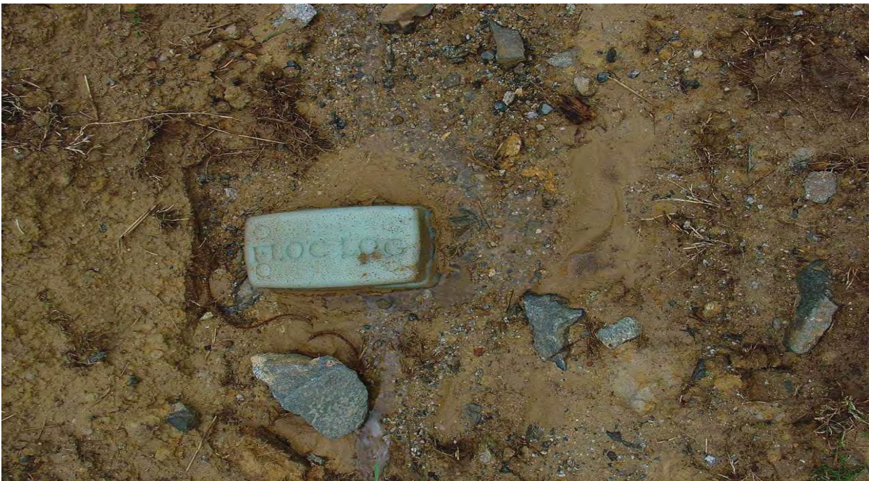
Flocculants are used to pull the finer particles out of the water to reduce turbidity, and protect sensitive water resources.
