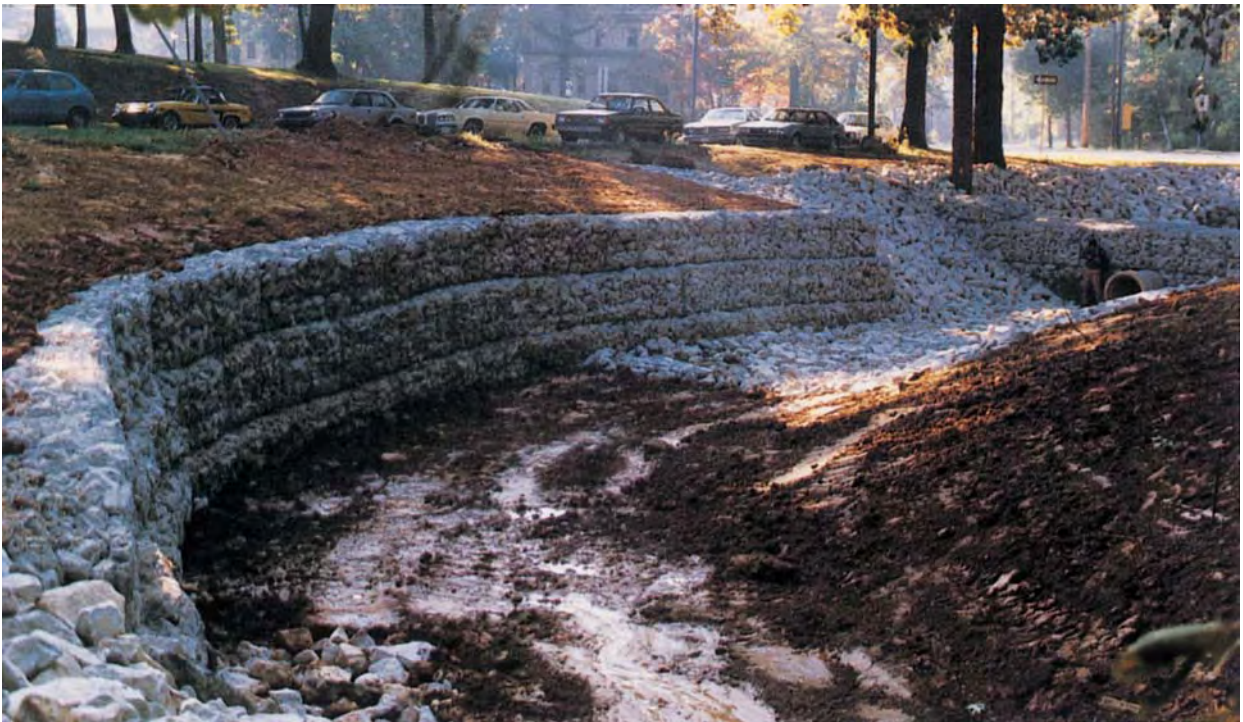
Structural streambank stabilization such as gabions and riprap is necessary where stream velocities are high and side slopes are steep.
