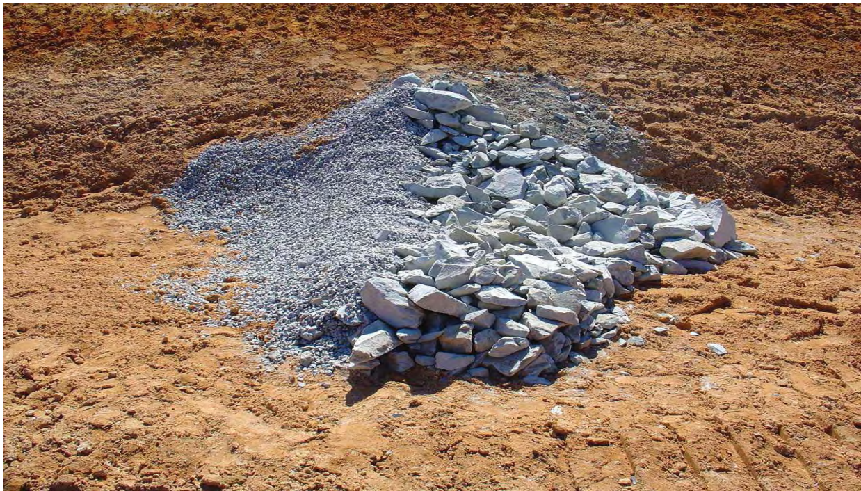
Check dams with weirs control the velocity of runoff through channels and reduce erosion.
