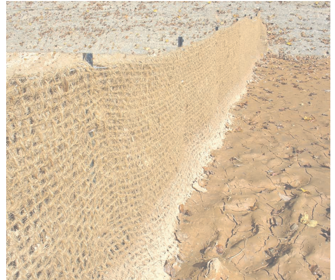
Figure 6.65d Close-up of a porous baffle.
