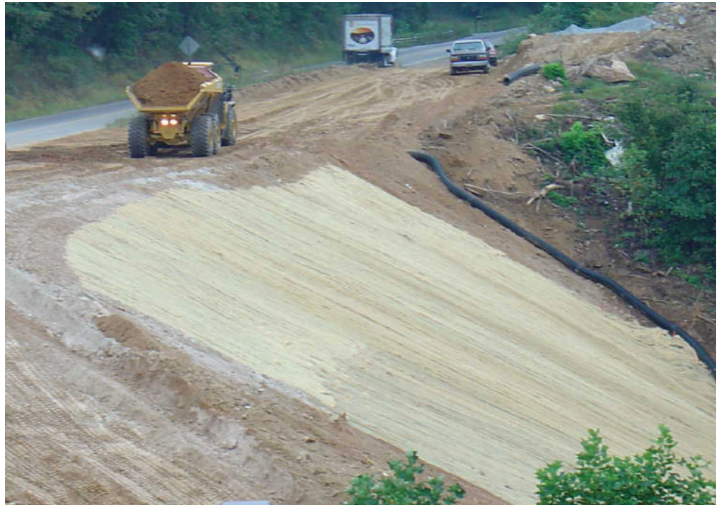
Rolled erosion control products hold seeds and mulch in place until vegetation is able to establish on steep slopes or channels.
