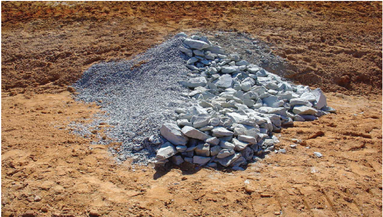
Check dams with weirs control the velocity of runoff through channels and reduce erosion.
