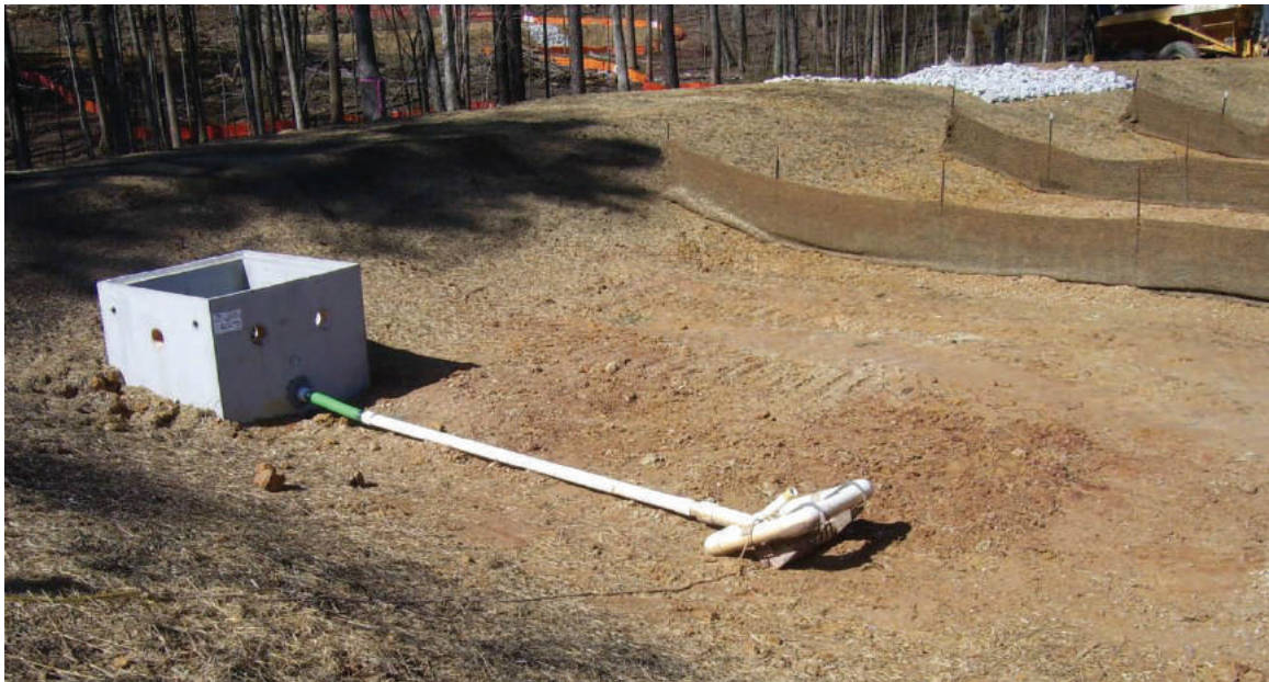
Figure 6.61b Sediment basin with skimmer attached to riser for dewatering. Photo Credit: Town of Apex
