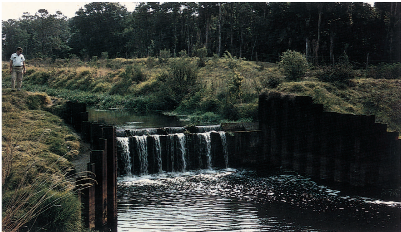
Grade stabilization structure prevents head cutting in a vegetated channel.
