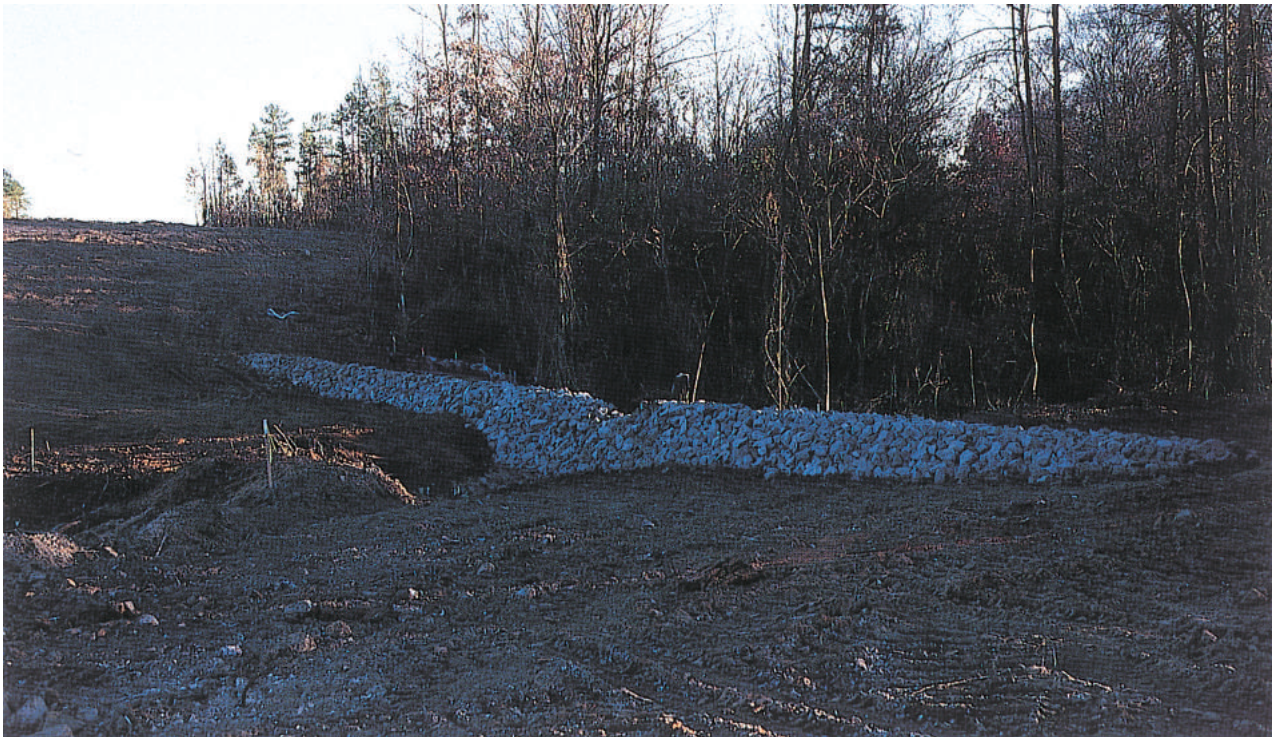
Rock dam forms a sedimentation basin with a broad-crested principal spillway to keep flow depth and discharge velocity low.
