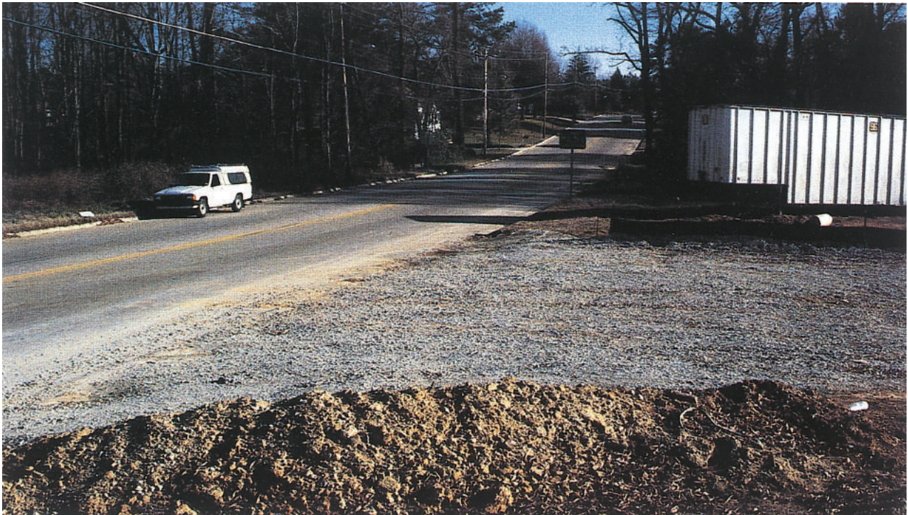
Construction entrance/exit provides an immediate buffer for on-site deposition of mud and sediment.
