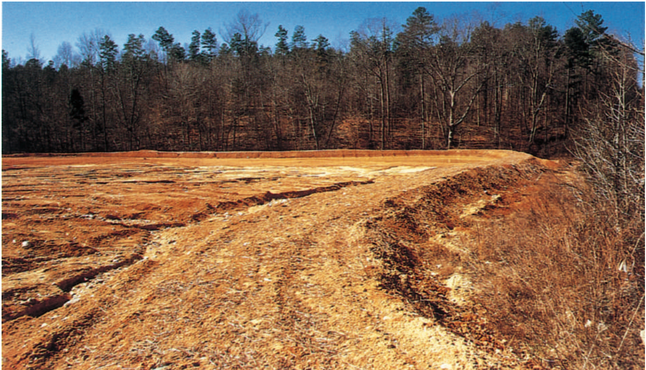
Diversion dike protects work areas and prevents sediment from leaving the site.
