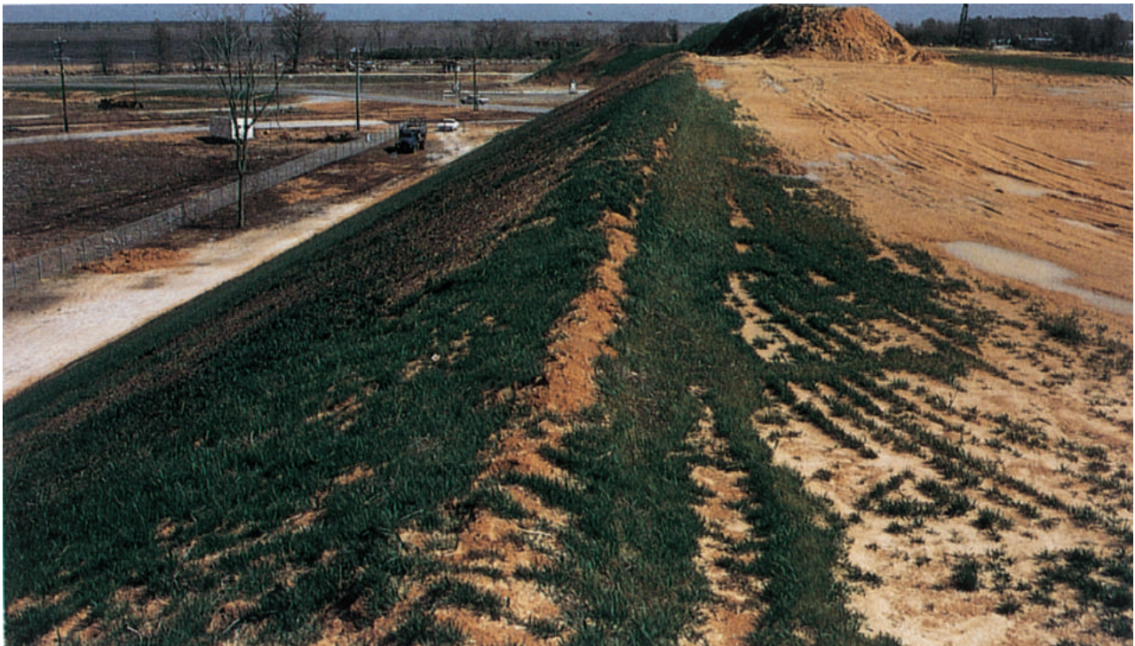
Permanent diversion controls the direction and velocity of runoff for erosion control and flood protection.
