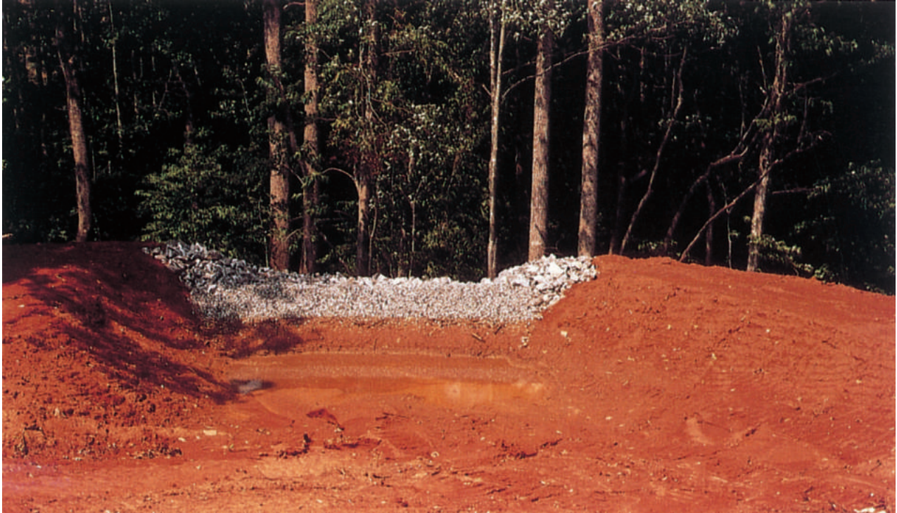
Temporary sediment trap provides a settling pool for a small drainage area. Gravel allows dewatering and a stable outlet.
