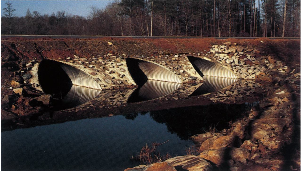
Permanent stream crossings require structures that will not erode, overtop, or cause flooding.
