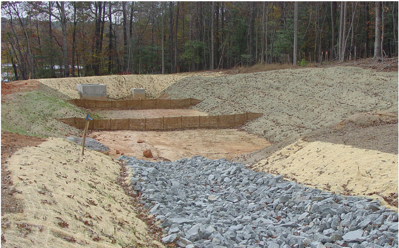
Sediment basins are strategically located to trap sediment near the outlet of a work site.
