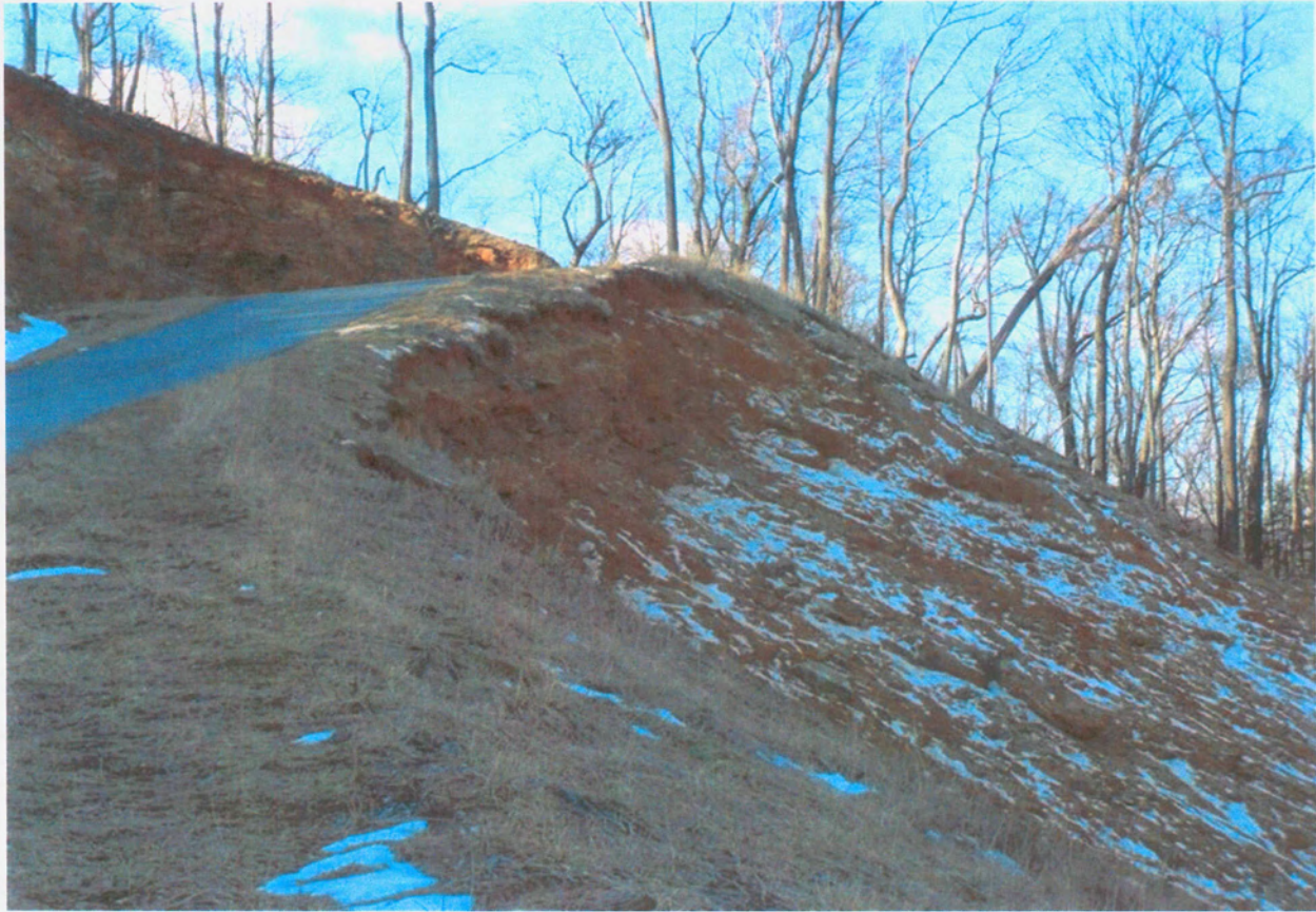
Failing Cut and Fill Slopes at Chocolate Drop Mountain, Polk County
