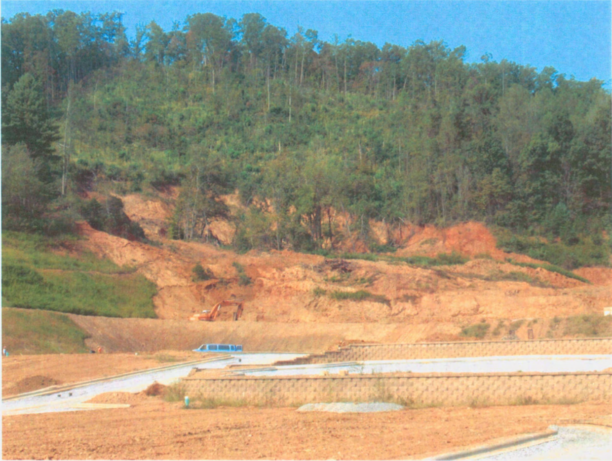
Macon County slide. Trees standing in center of slide actually slid 30-50 feet down slope from original location.
