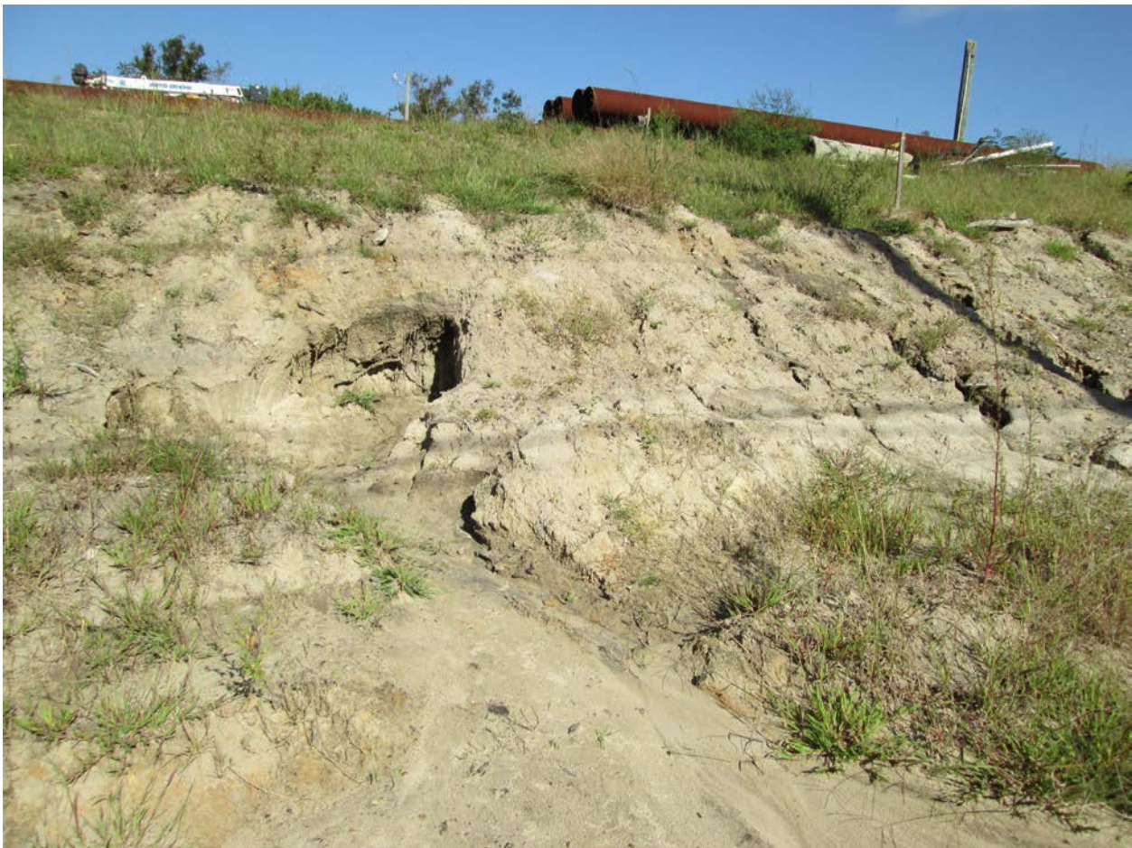
Eroding Slope, Piney Green Road
