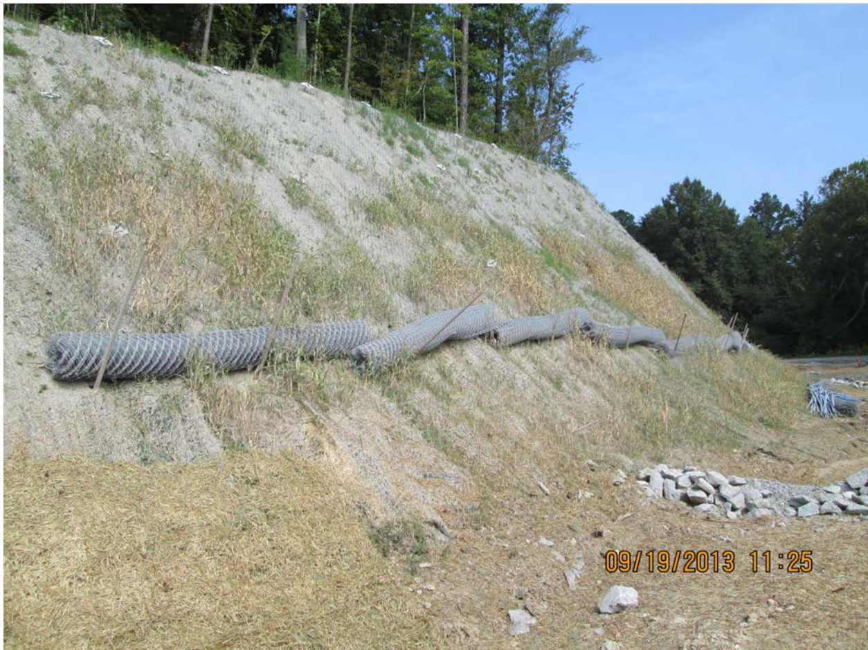
Howard Gap Road, SR 1006—Cut slope being stabilized with soil anchors and chain link fence over seeding and matting.
