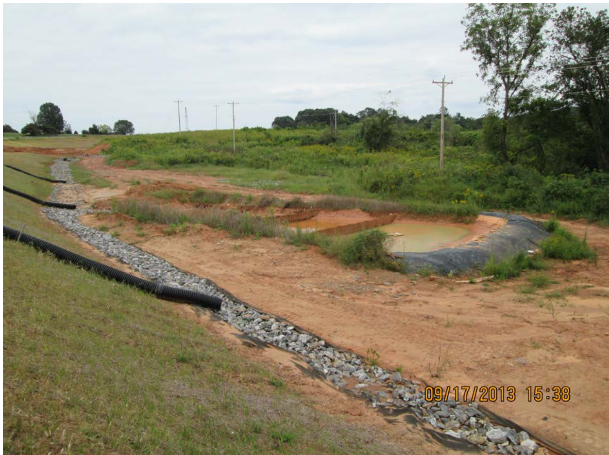
I-40 and I-77 Interchange—Area above and below skimmer basin needed ground cover.
