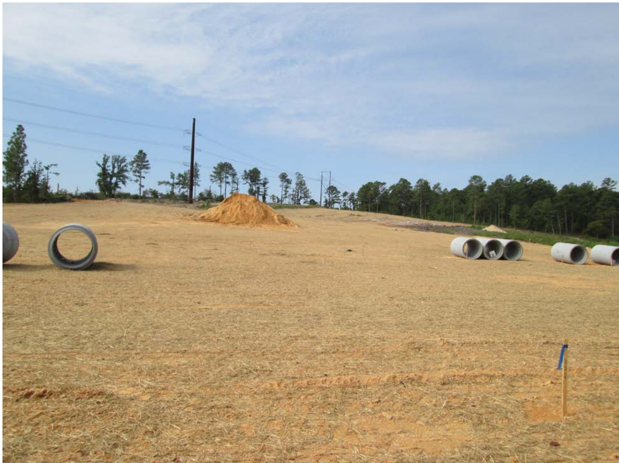
Large exposed area not draining to a sediment basin, Fayetteville Outer Loop
