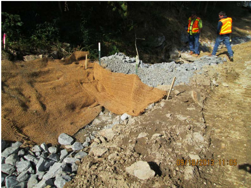
Big Branch Road, SR 1156— Left, Riprap lined ditch and check dam above culvert inlet.
