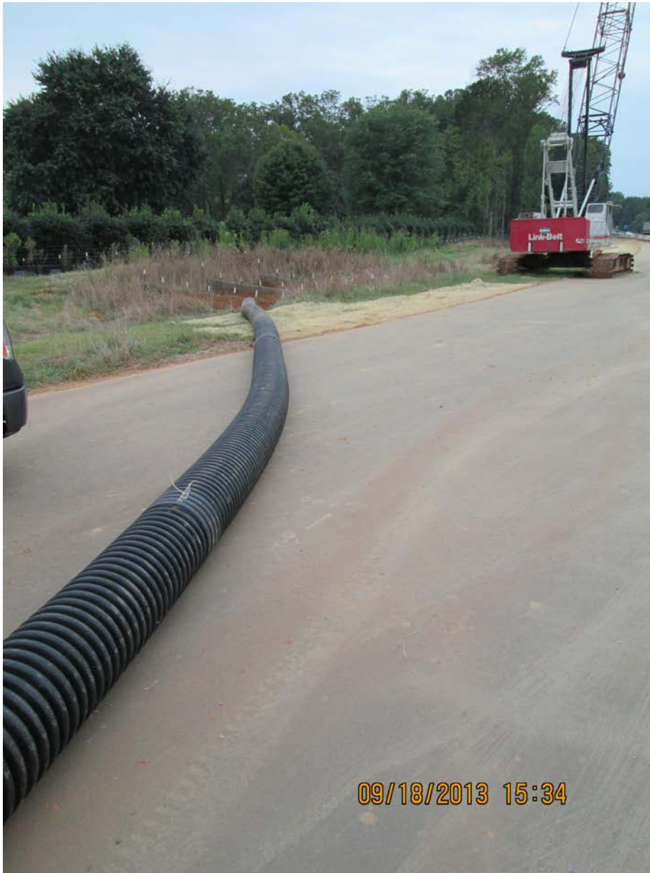
SR1922 and SR 1924— Slope drain conveying runoff from I-40 across new ramp to skimmer basin.
