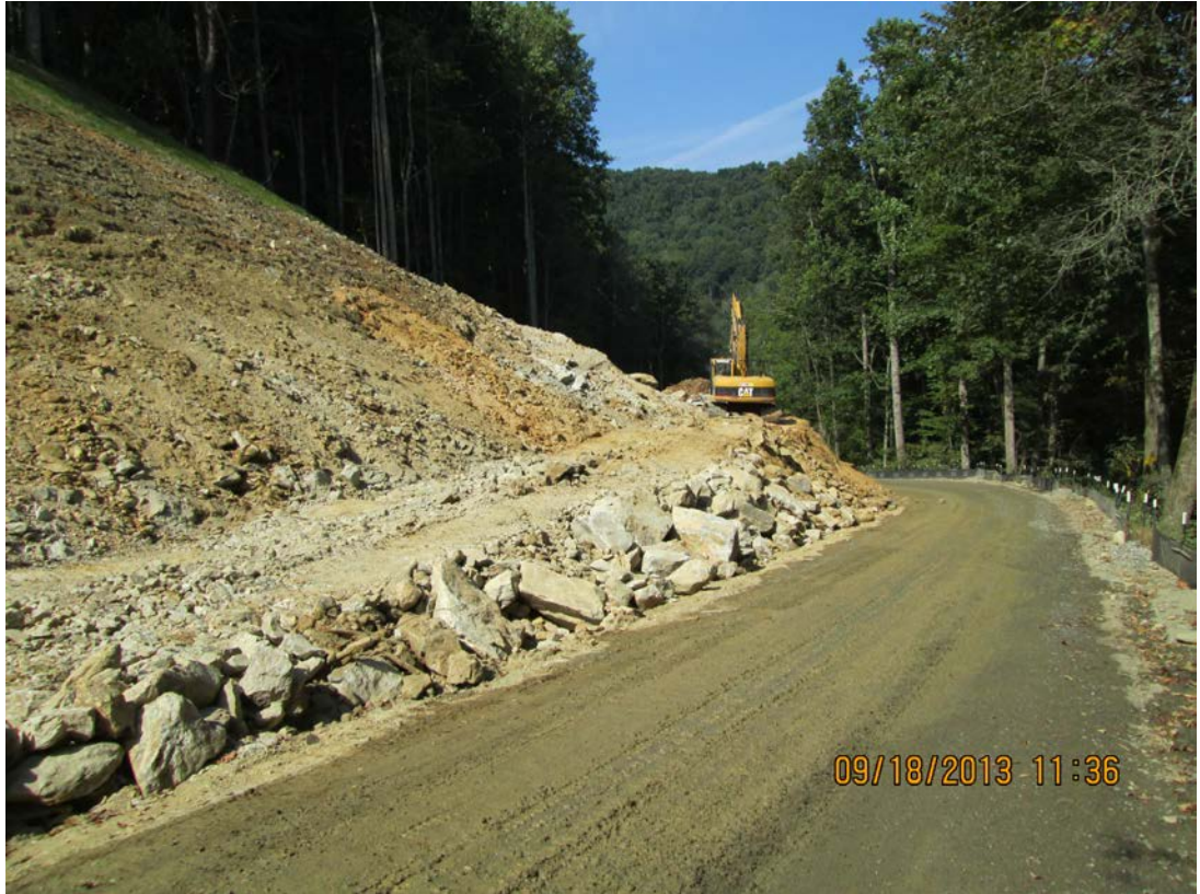
Big Branch Road, SR 1156— Right, cut slope being graded with seeding on upper slope.
