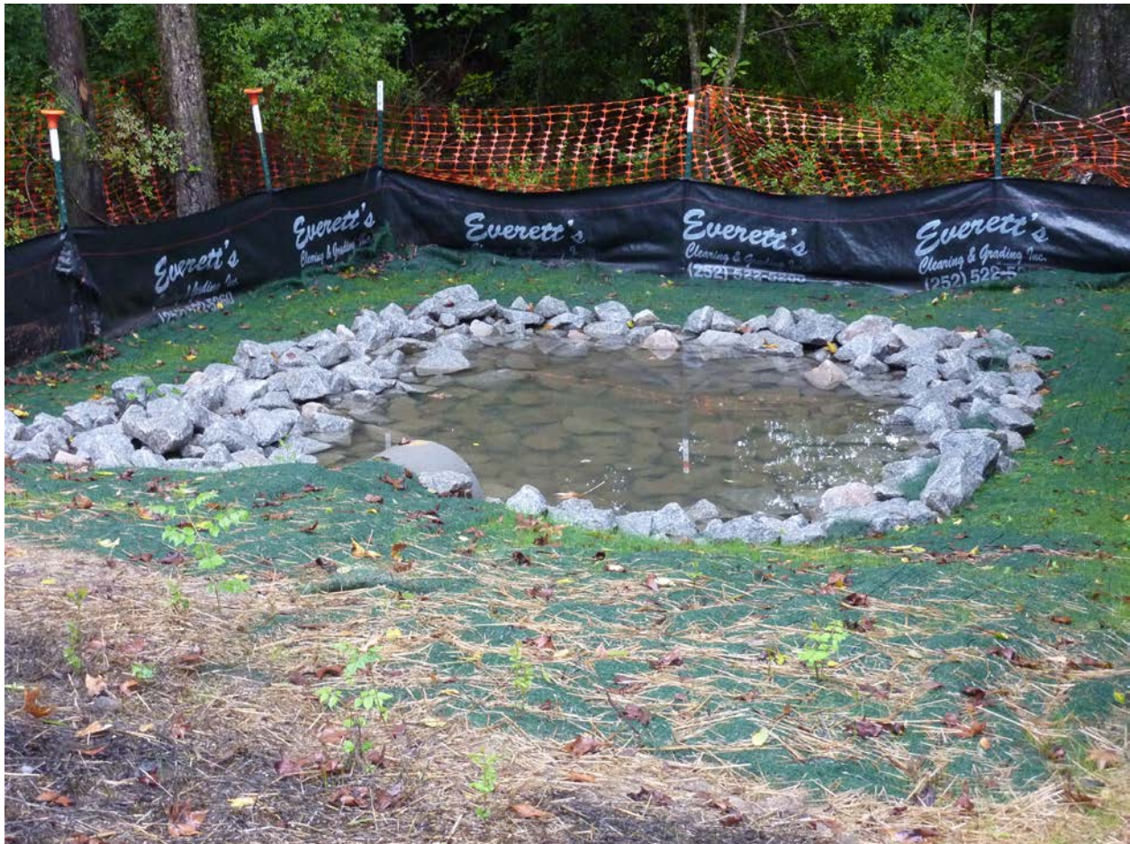
Scour Hole, Pitt County Bridge Replacement
