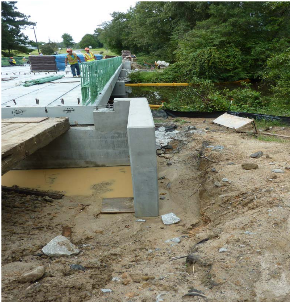
Unstabilized areas around wingwalls, Bridge 201 Over Little River
