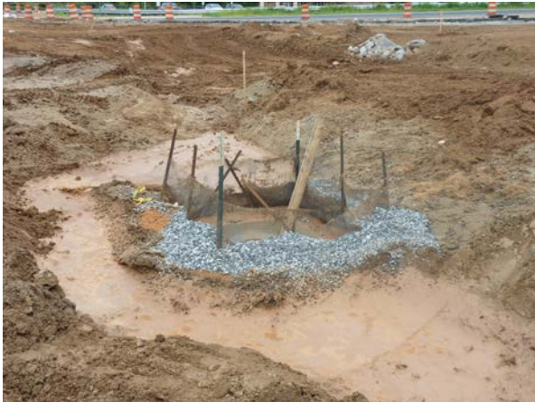
NC-18 and I-40 Interchange—Inlet in Need of Maintenance
