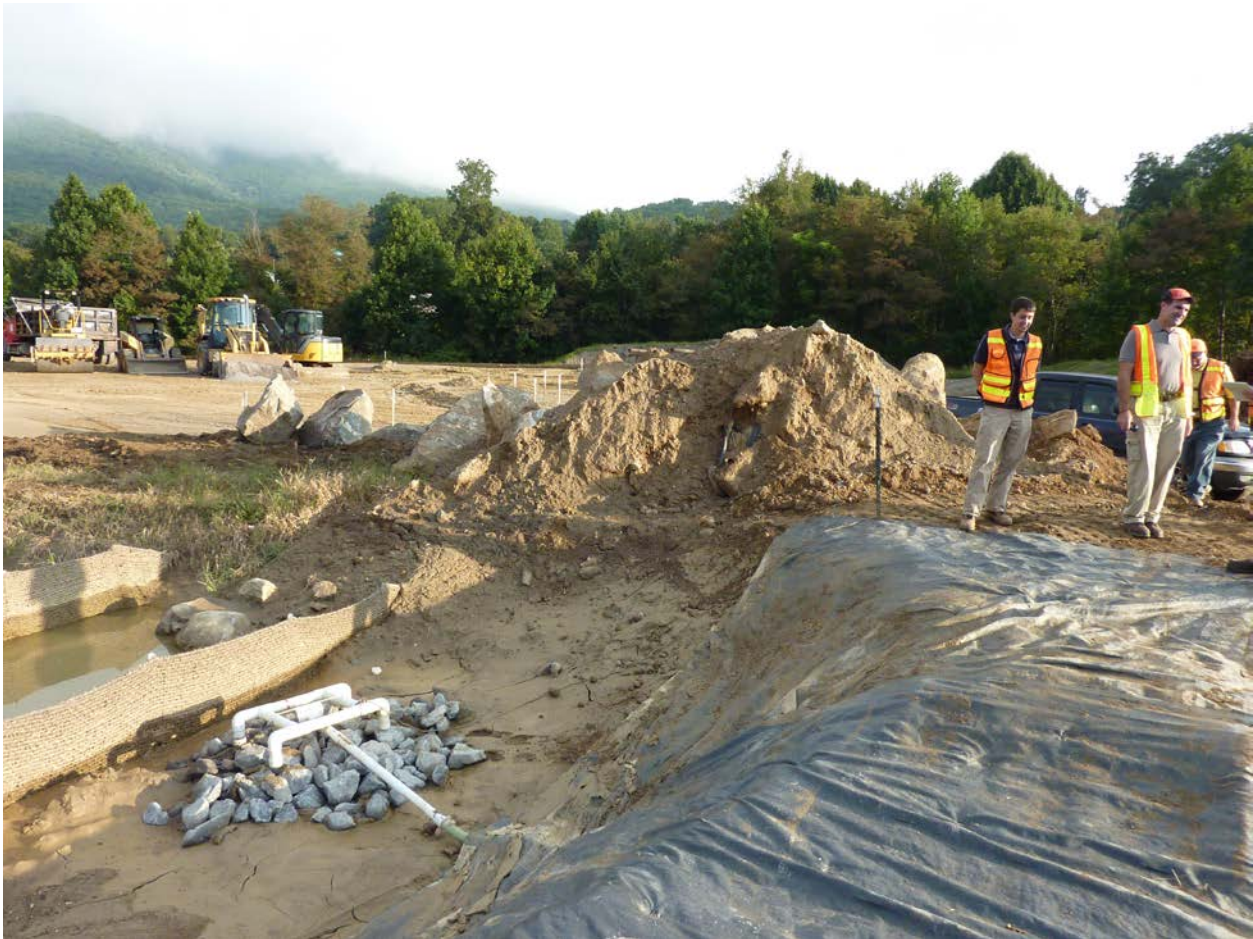
Rock/Dirt Pile at Outlet of Skimmer Basin, US 23/74 Southbound Rest Area
