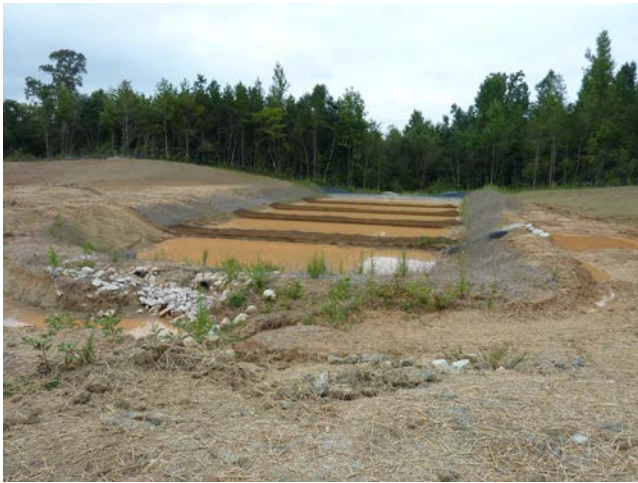
Skimmer Basin at Borrow Pit; Below, Turbid Water at Skimmer Basin Outlet
