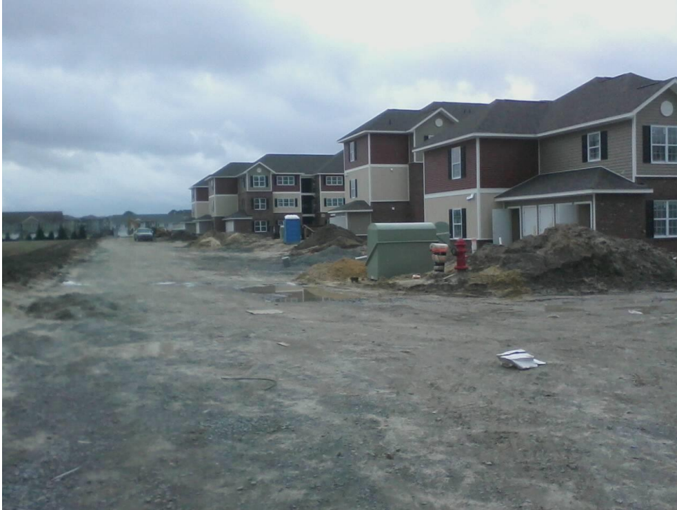
Kittrell Place - Soil stockpiles and perimeter berm (on left) should be vegetated.
