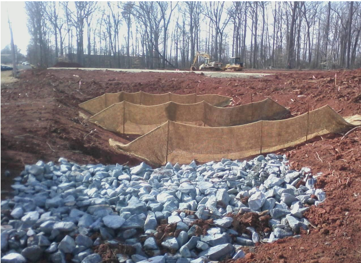
Dollar General – Basin installed was smaller than that called for on approved plans.
