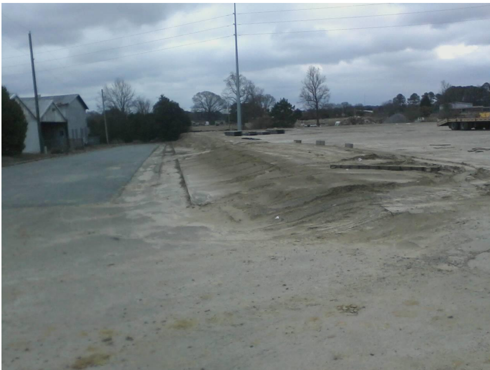
Save A Lot – Additional unpermitted disturbed footprint on right sloping to street lacks sufficient sediment controls. Sediment observed in downstream storm drain.
