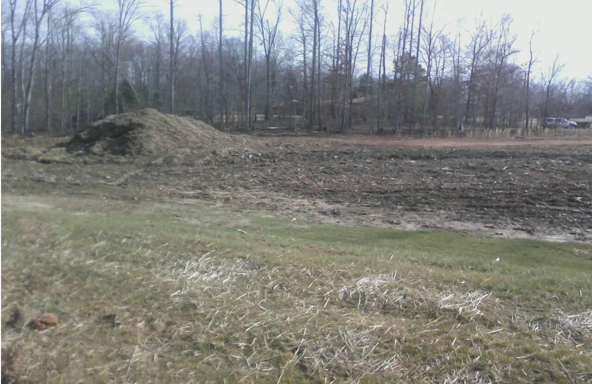
Big Boy Solar Farm – Denuded area beyond previously approved limits of disturbance.
