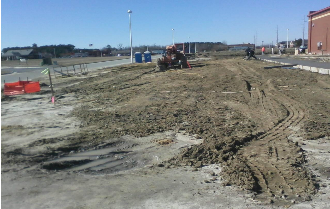
Lemongrass Restaurant – Perimeter silt fence removed prematurely. Fabric inlet protection utilized instead of hardware cloth and gravel. Deposition on Fire Tower Road.
