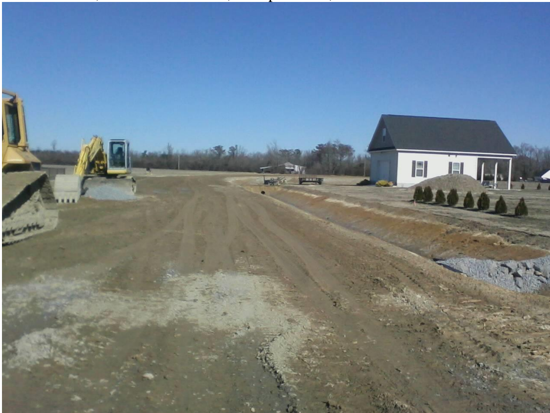
Oak Pointe - Roadside ditches have check dams but no groundcover.
