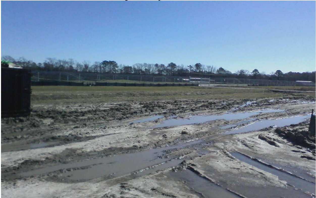
Rams Horn Solar Farm – Silt fence remaining until dense stand of permanent vegetation is established.
