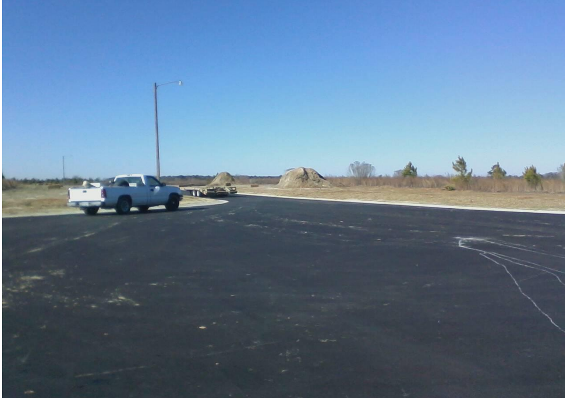
Whitaker Glen, Section 2 – Ditches, stockpile areas, and other areas on site are bare.
