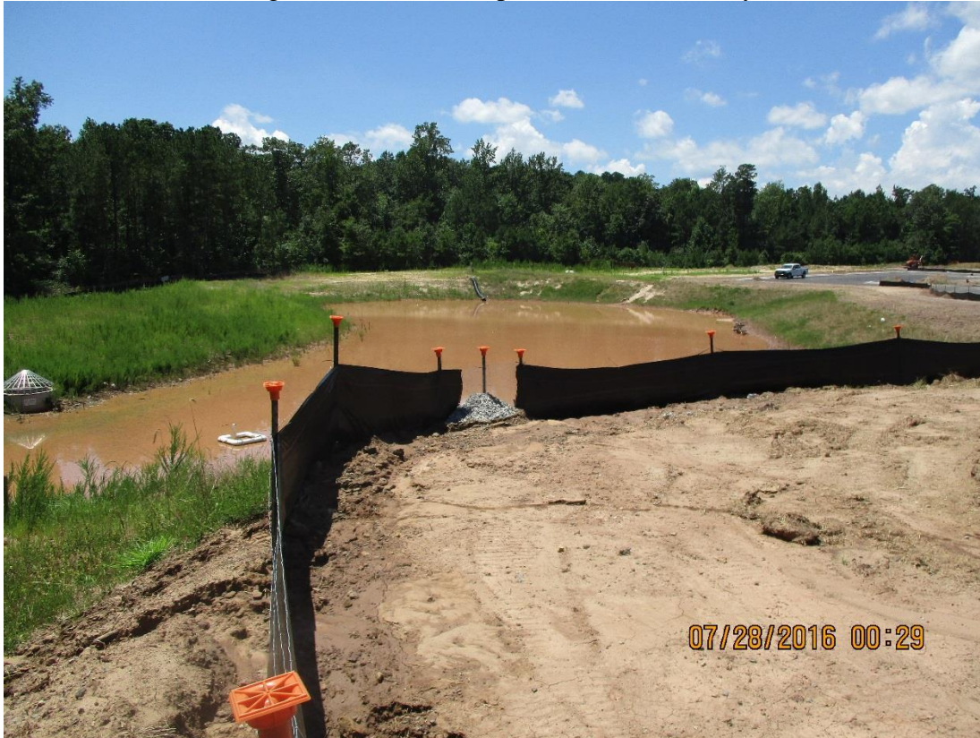
Site 2 – Silt fence undermined causing erosion on downstream slope.
