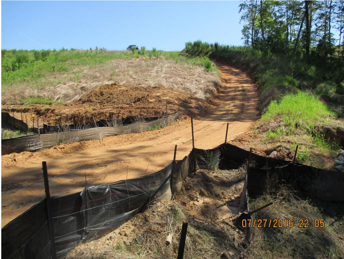
Site 1 – Stream crossing needs additional upstream runoff conveyance and sediment storage.
