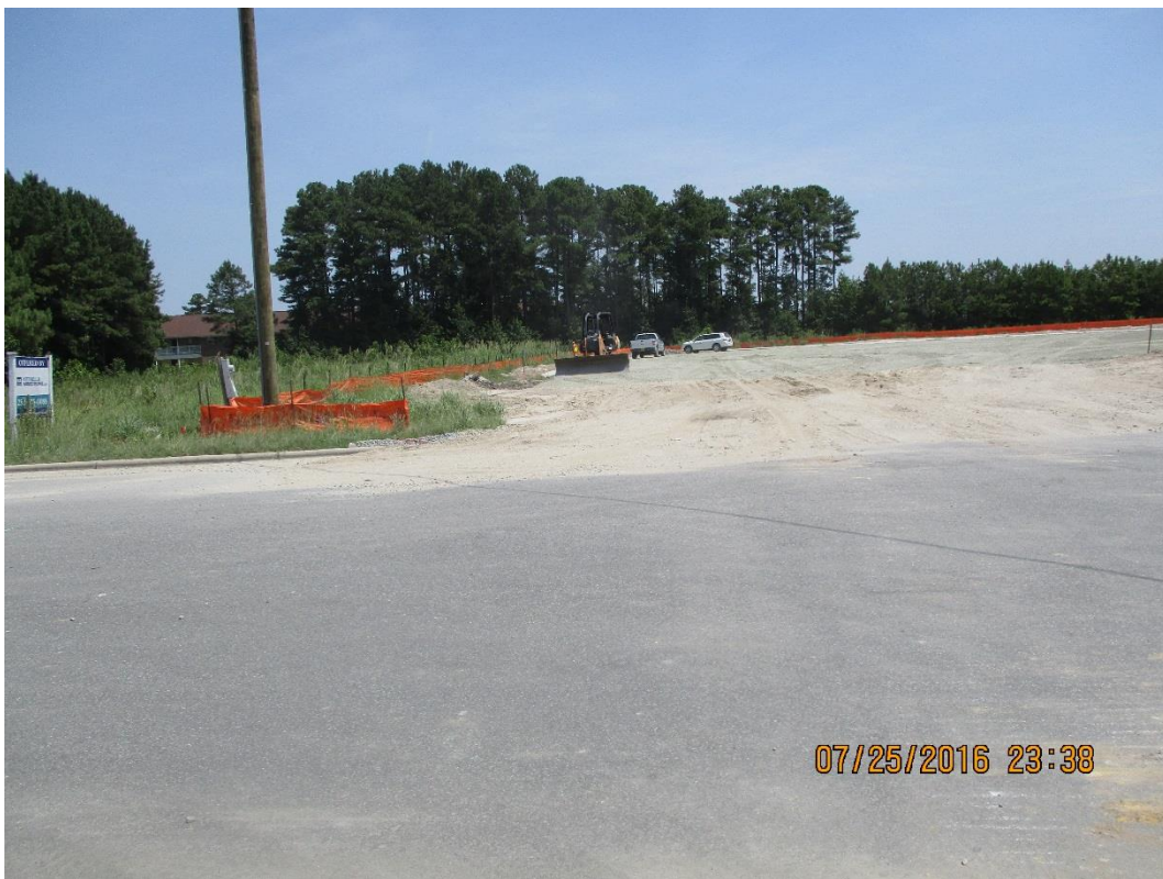
Site 2 – Sediment in street at construction entrance.
