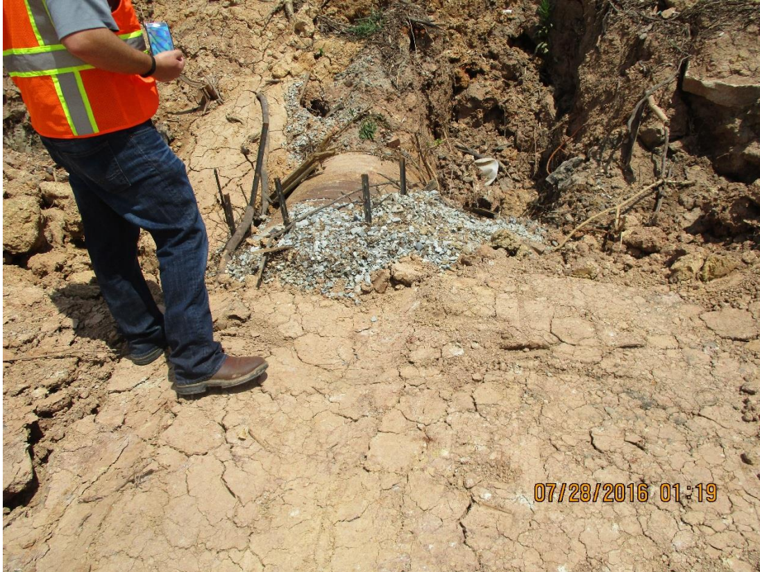
Site 3 – Inlet protection blocked with compacted fill.
