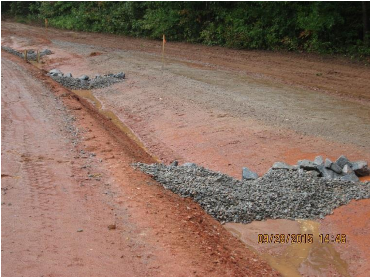
Erosion and sedimentation in roadside ditch
