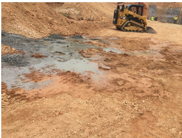
Figure 1 - Unmanaged Concrete Washout Area
