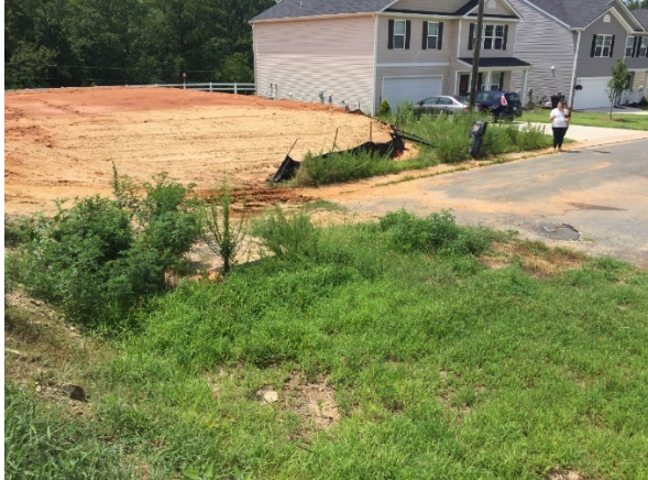
Figure 3 - Poor Practice - No Construction Entrance
