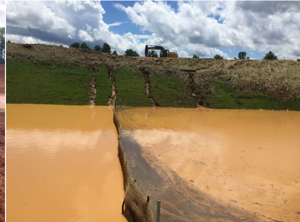
Figure 6 - Rill Erosion on side slope of the Sediment Basin
