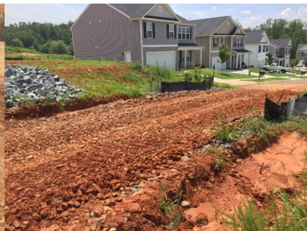
Figure 2 - Construction Entrance needs maintenance
