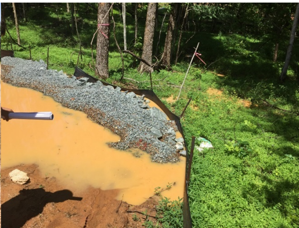
Figure 8 - Silt Fence Outlet in Wrong Location
