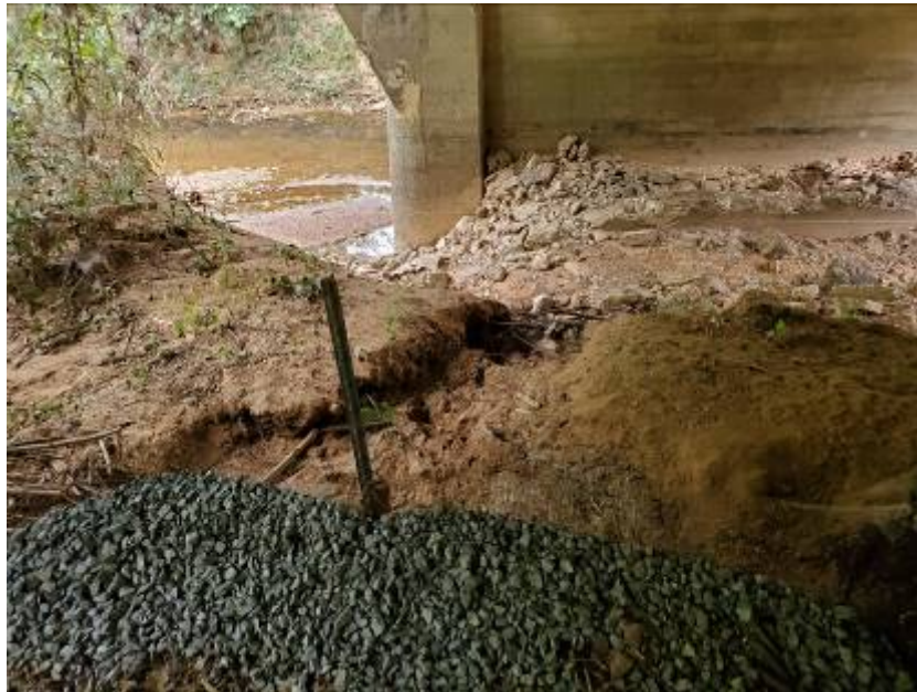
Photo - Gully erosion beyond silt fence outlet. (9/5/2019)
