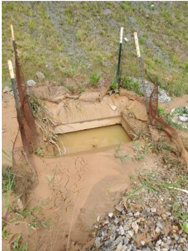
Photo - Unmaintained inlet protection full of sediment and water. (6/25/2019)
