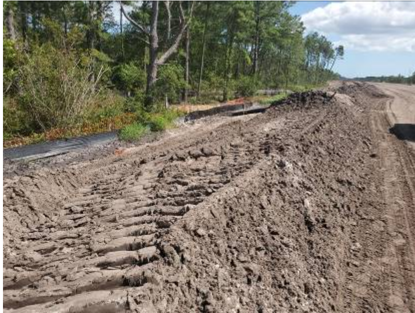
Photo - Location of offsite sedimentation post large rain event. (8/27/2019)
