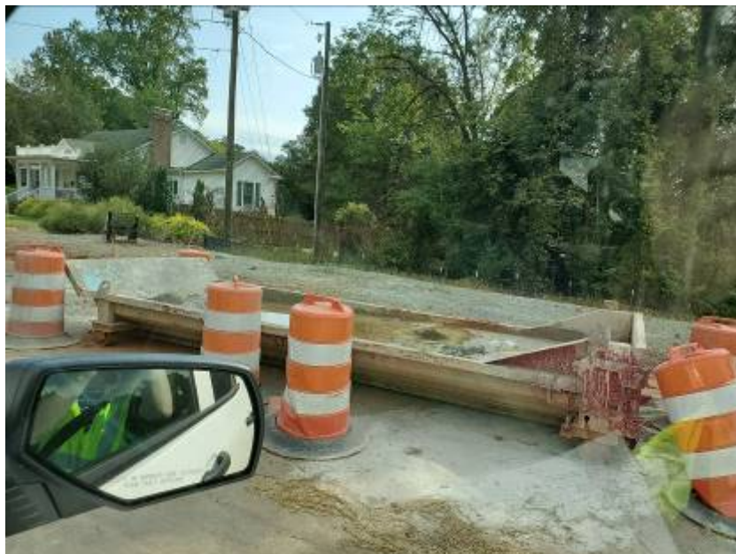
Photo - Concrete washout with no secondary containment. (9/18/19)
