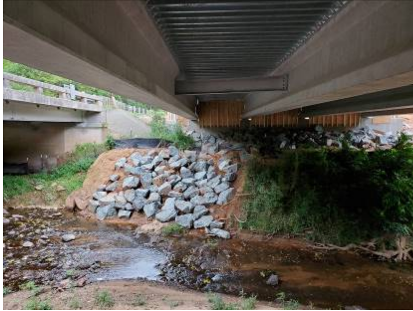
Photo - Slope failure temporarily stabilized with rock. (9/5/2019)
