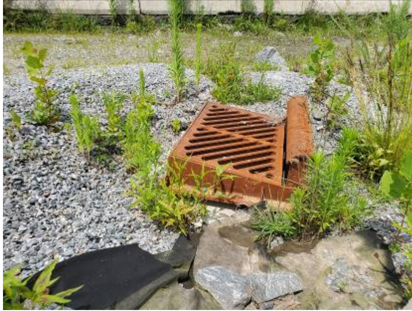
Photo - Poorly protected inlet. (6/25/2019)
