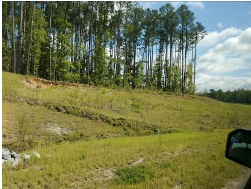
Photo - Slope Failure. (8/28/2019)
