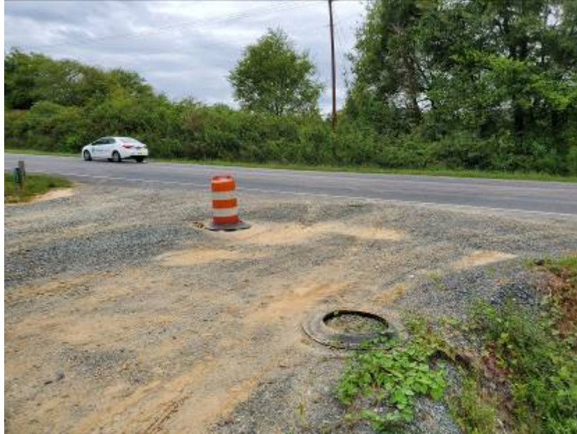
Photo - Construction entrance needs to be freshened up. (9/5/2019)
