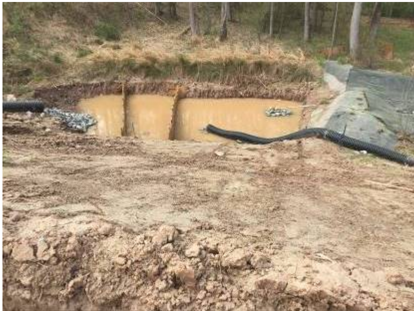
Photo - Skimmer basin with damaged liner and no bank stabilization. (4/5/2019)
