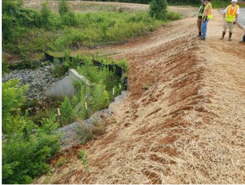
Photo - Slope above permitted creek needing more groundcover. (6/25/2019)
