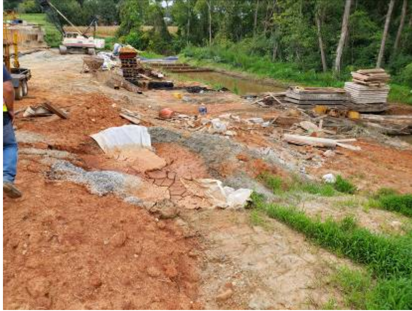
Photo - Construction debris and unmaintained concrete washout. (9/5/2019)
