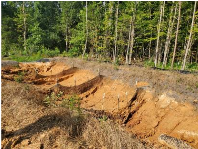
Photo - Recently mucked basin in need for baffles to be replaced. (8/7/2019)
