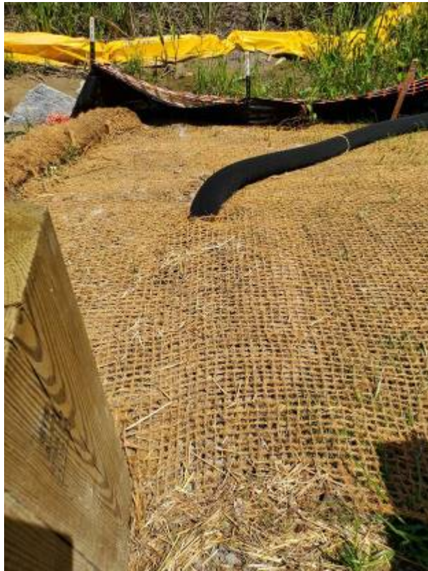
Photo - Undersized slope drain. Rill erosion underneath mat. (5/16/19)
