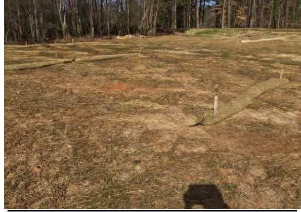
2. Area where matting may need to be installed to establish ground cover.
