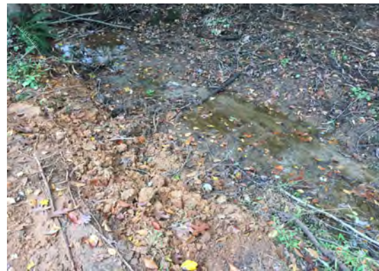
4. Damage to unclassified stream on site.
