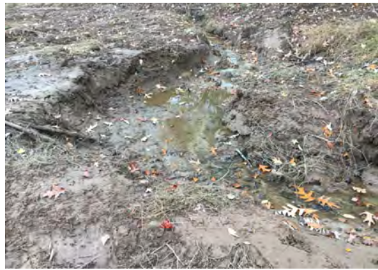
6. Damage to unclassified stream on site.
