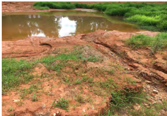
3. Repair erosion around pond and stabilize.
