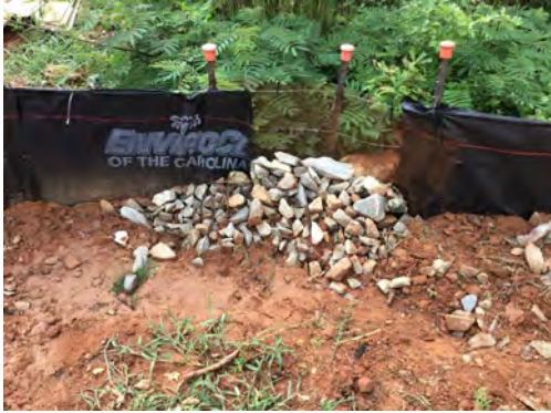
Comment: lot 16, silt fence outlet needs 57 stone
