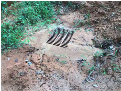
Comment: inlet protection needed behind lots 88-90
