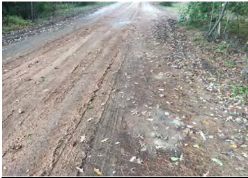
7. Mud tracked onto road
