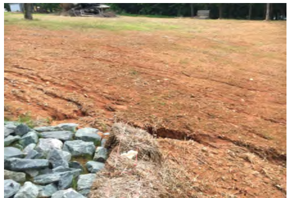
4. Repair erosion around rip rap. Ensure lowest point is in the middle of the rip rap.
