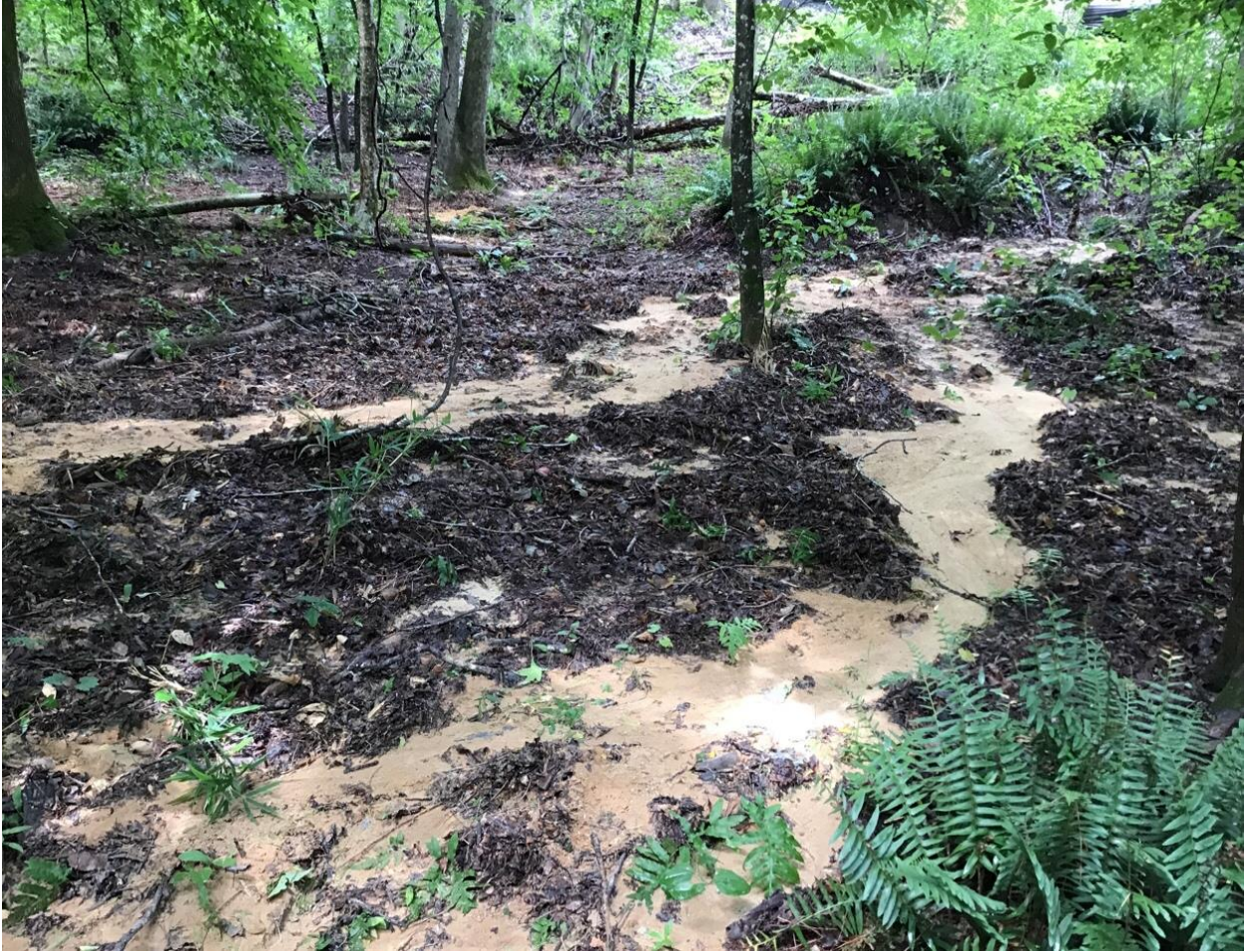
Comment: Miller Stone Rd. - sediment in riparian buffer
