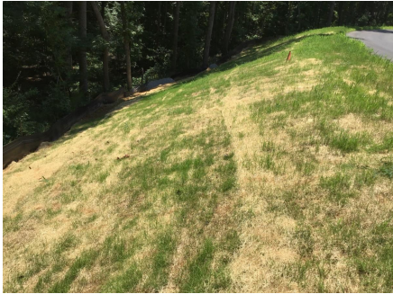
Comment: Slope stabilized
