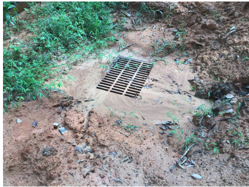
Comment: inlet protection needed behind lots 88-90
