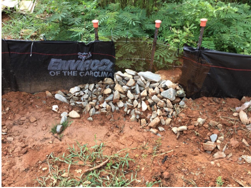
Comment: lot 16, silt fence outlet needs 57 stone
