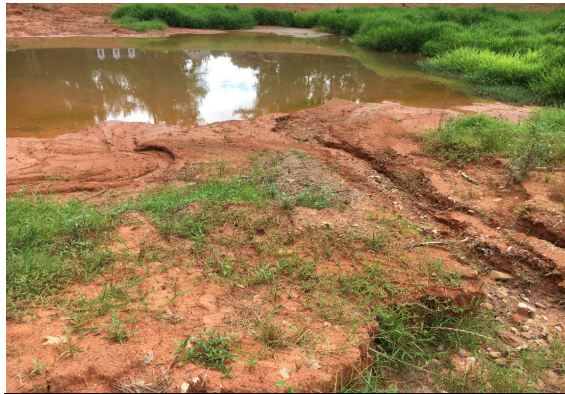
3. Repair erosion around pond and stabilize.
