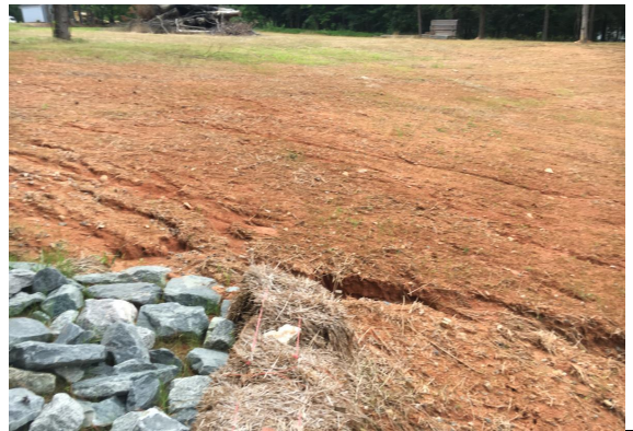
4. Repair erosion around rip rap. Ensure lowest point is in the middle of the rip rap.
